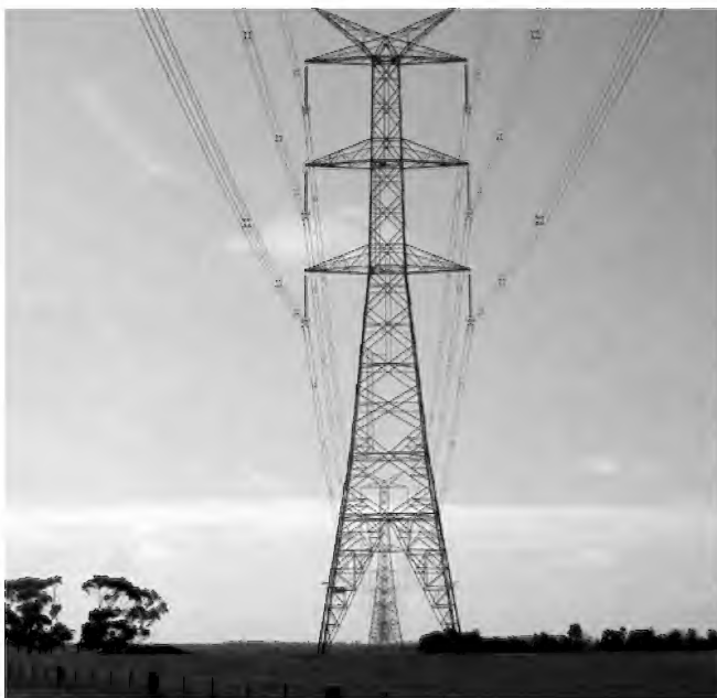
Moving energy across large landscapes: power line towers stretched across the Basalt Plain near Cressy Victoria.
