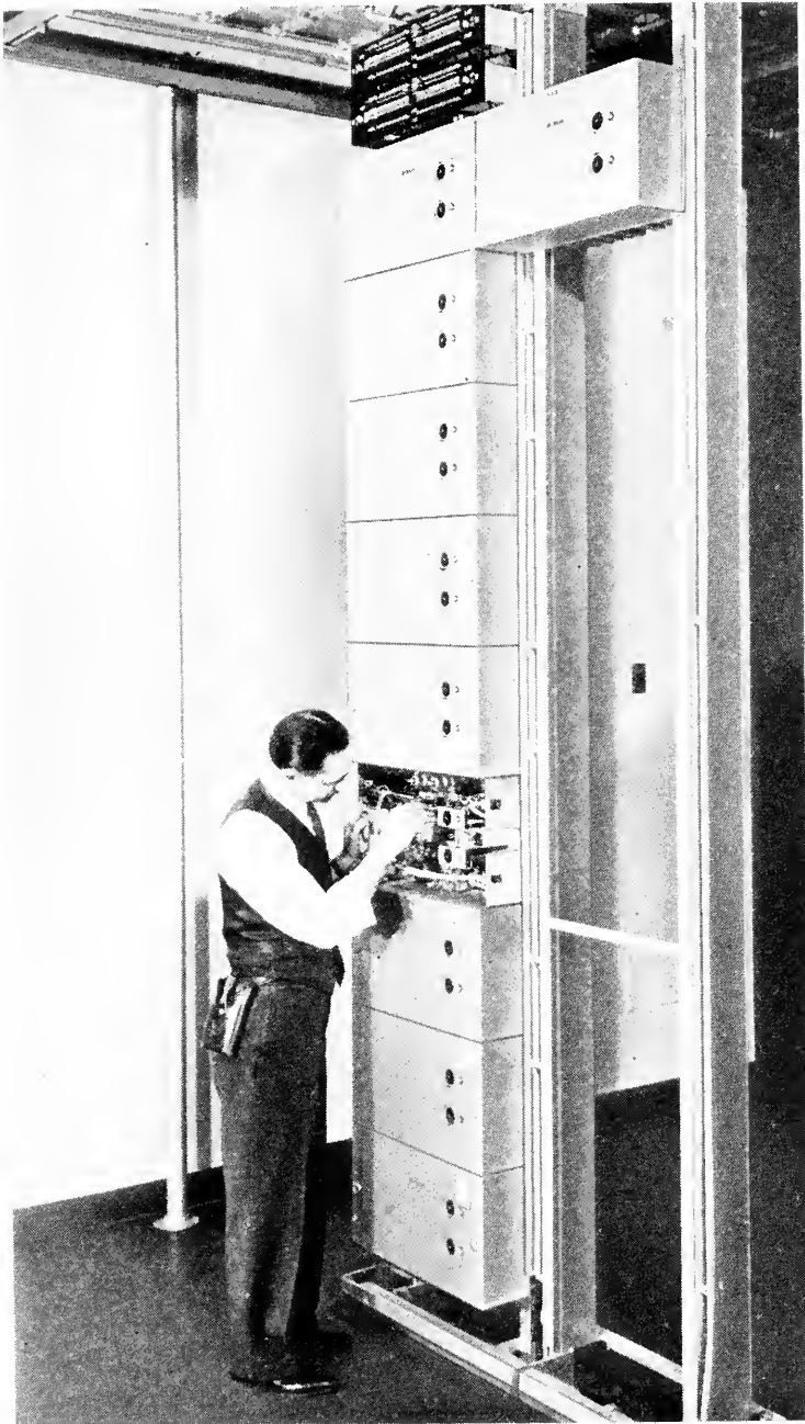
Fig. 13—Bay arrangement for group modem equipment as installed at New York.
