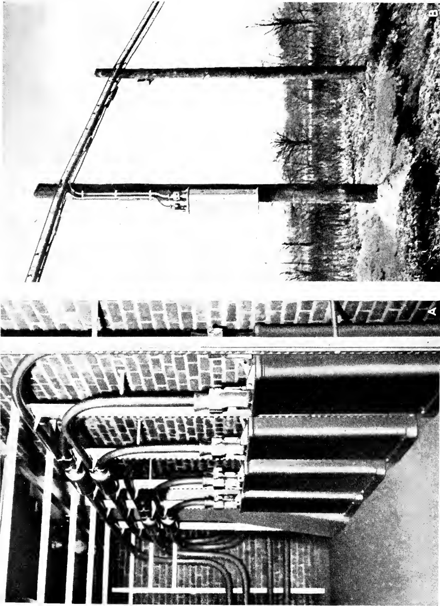
Fig. 7-A—Retardation coil cases installed in cable vault at West Unity, Ohio.
