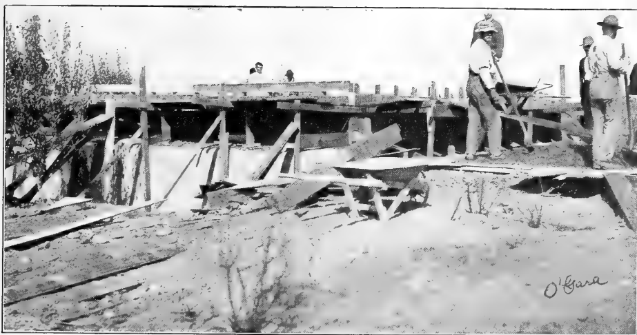
Crude Oil Tank in Palmer Investment Company's Orchard, Medford, Oregon
