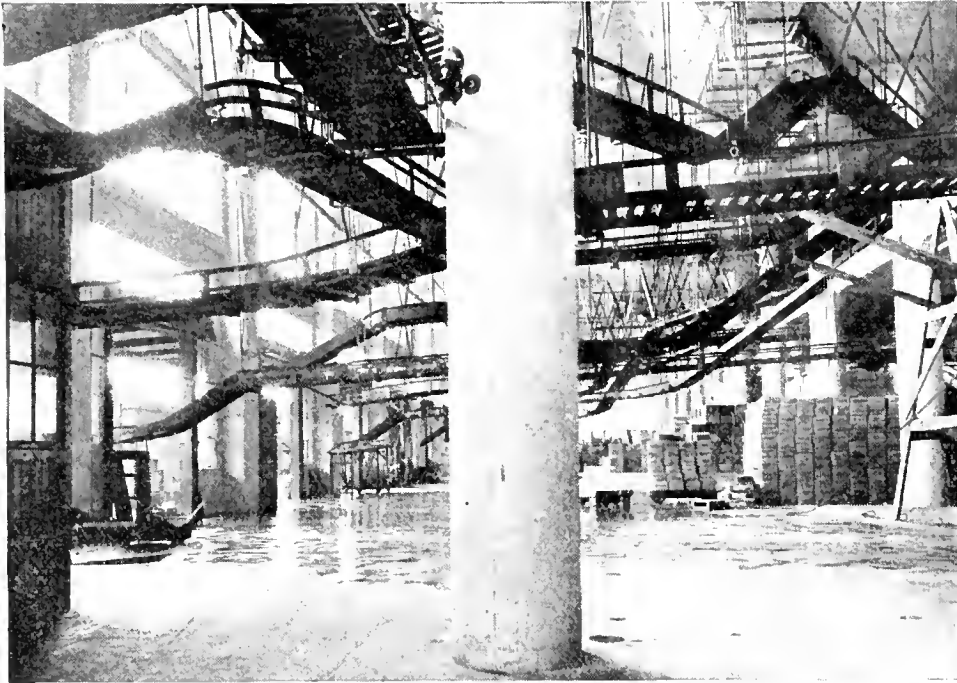
You may not require so pretentious a conveying system as that of the California Associated Raisin Company, shown above, but you can effect the same relative economy in your own establishment. (Note how the overhead system in this instance enables maximum utilization of floor space.)
