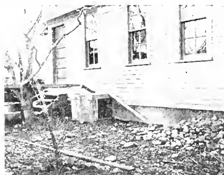
Air intake to a basement storage where the air duct is built on the outside. Such openings should be fitted with airtight doors and be located about fifteen feet apart on the sides and ends of the house.
