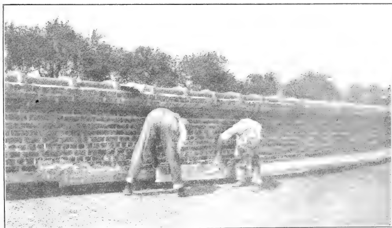
FIGURE 17.—Eaves of a tobacco warehouse sealed from the top of the building by pasting a strip of tough paper, 10 inches wide, over the flashing where it joins the brick wall.
