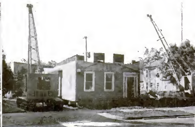
4. UNROOFED FIRST FLOOR, with part of second story also gone, is moved in conventional way.
