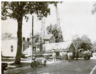
3. CRANES MOVE FORWARD and lower attic and roof section onto body of flatbed trailer.
