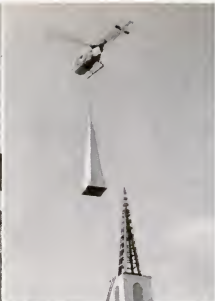
2. STEEPLE ALOFT makes pass at tower frame. Third try nicks top, does no damage.
