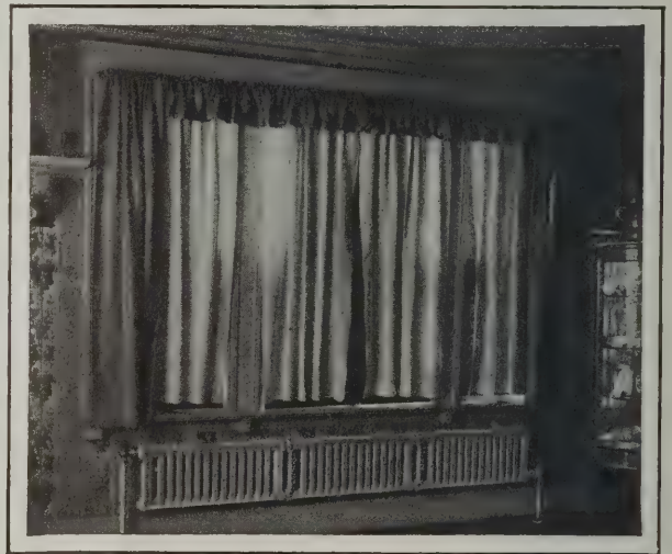
Fig. 4—Wall Radiator Under Window Valved for Modulation Heating
