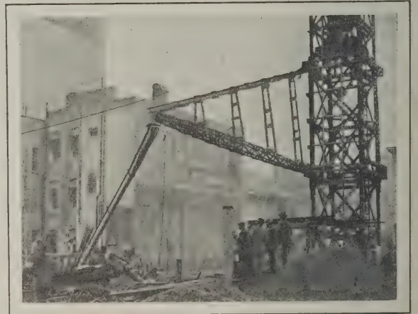
Fig. 11—A Convenient Method of Distributing and Placing Concrete in the "Forms" on a Building in Progress of Erection
