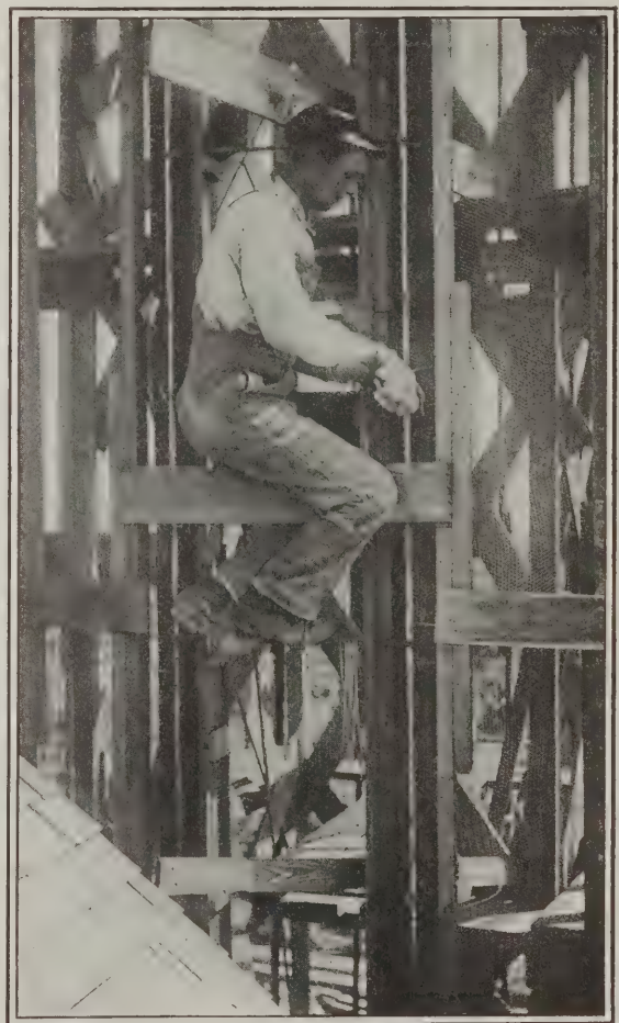
Fig. 2—Showing Method of Placing Reinforcing Material in the "Forms" for the Door Posts
