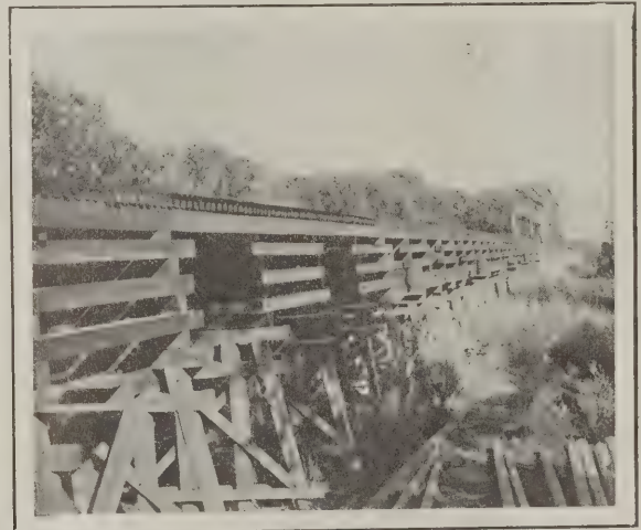
Fig. 2—Method of Cribbing on Top of the Original Bents of the Trestle
