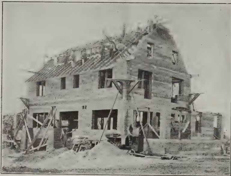
Van Guilder System of Hollow Wall Construction—Fig. 9—Showing a Machine in Use at Top of End Gable
