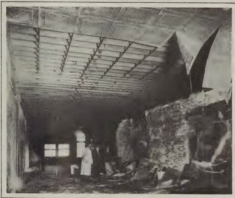
Metal Ceiling as a Fire Retardant—Interior of Garage After Fire Showing Protection Afforded by Metal Ceiling
