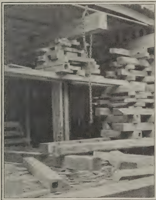
Fig. 4.—A Detail Showing the Manner of Removing the Beams used as "Needles"
