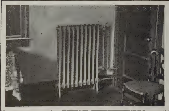
Modulation Heating of a Residence. Fig. 2—Radiator with High Legs for Bedroom—Water Seal Motor Valve is in Closet and on Same End as Modulation Valve
