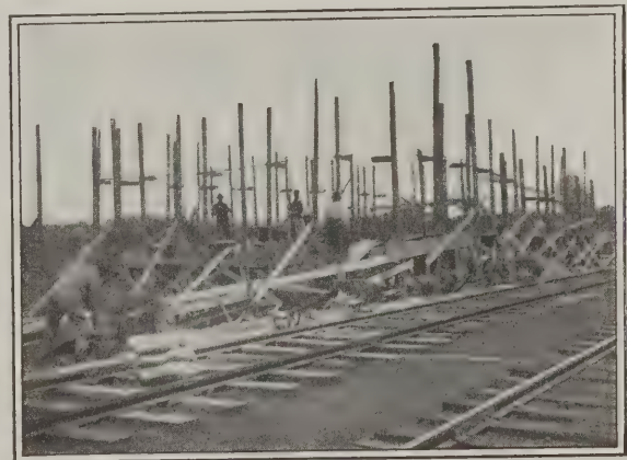
Method of Conveying Concrete to "Forms" and Showing Water Supply Hose Under Railroad Track
