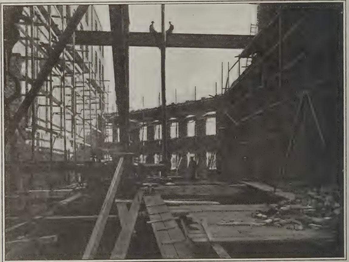
View of the Bank Building in Progress of Erection and Showing the Steel Girders Being Placed in Position
