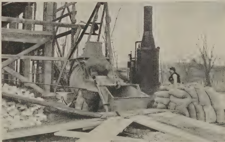
Concrete Construction in the Winter—Fig. 1 Showing One Method of Heating Water by Means of Steam
