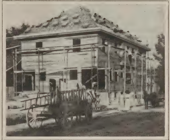
Fig. 7—Manner in Which Bundles of Shingles Were Distributed Over the Roof Area
