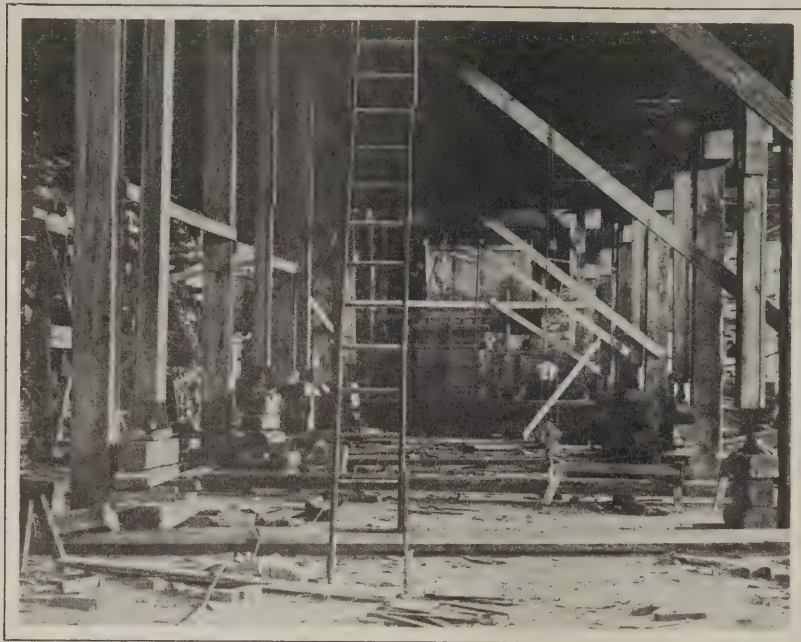
How a Large Truss Roof Was Raised—Fig. 5—Manner of "Loading" the Roof on the Screws
