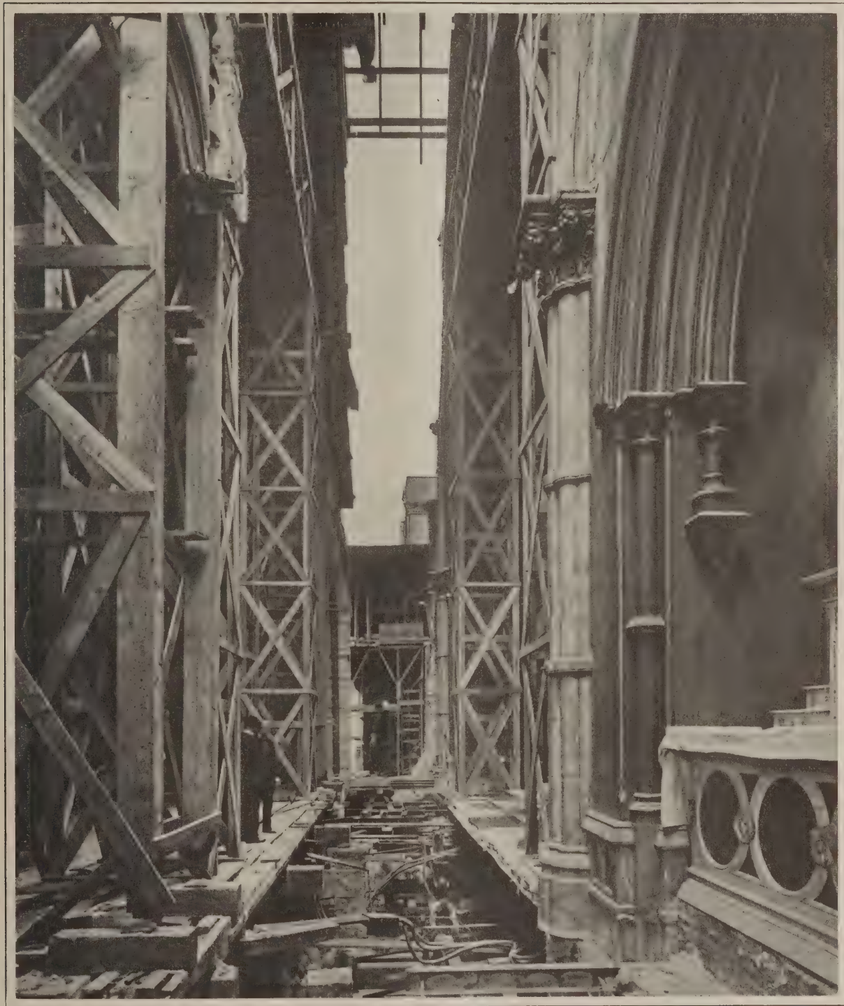
A Notable Church Remodeling Operation—An Inside View Showing the Sections After the Removal Had Been Completed
