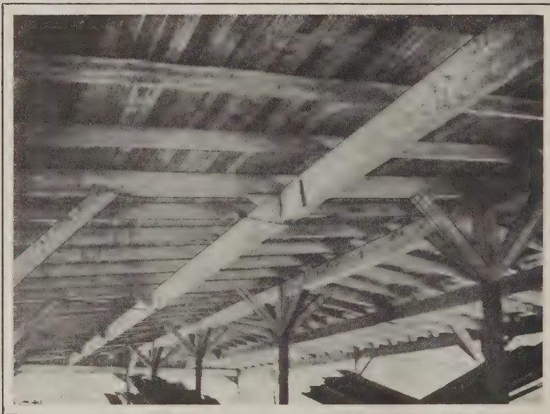
Partial View of Under Side of Shed Roof Showing the General Arrangement of the Framing Members
