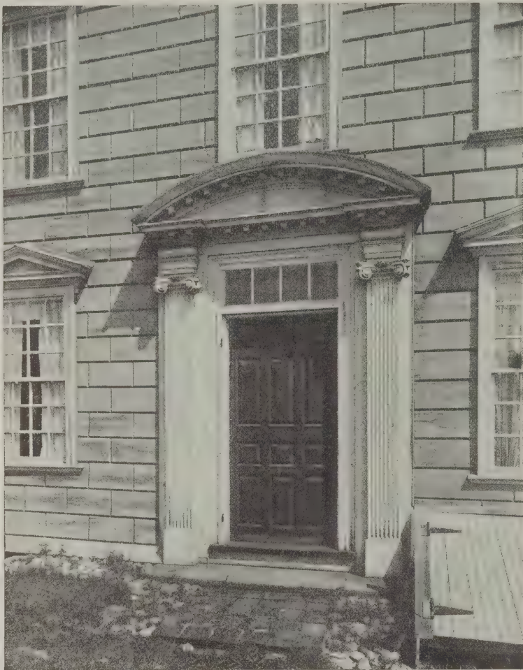
DOORWAY, ISAAC ROYALL HOUSE at Medford, Massachusetts. Built of White Pine in 1732.
