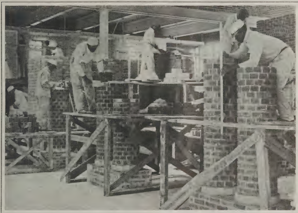
Industrial Education in the South—Fig. 8—Students of the Class in Bricklaying at Work—This Is One of 13 Trades Taught Boys at Hampton Institute Trade School
