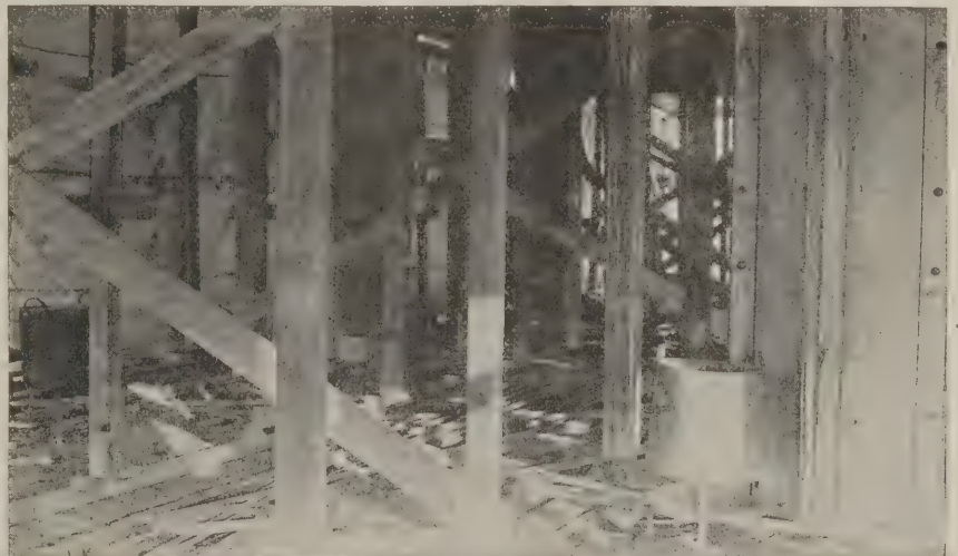
Fig. 3—Showing Use of Salamanders for Keeping the Enclosed Work During the Process of Construction at the Proper Temperature
