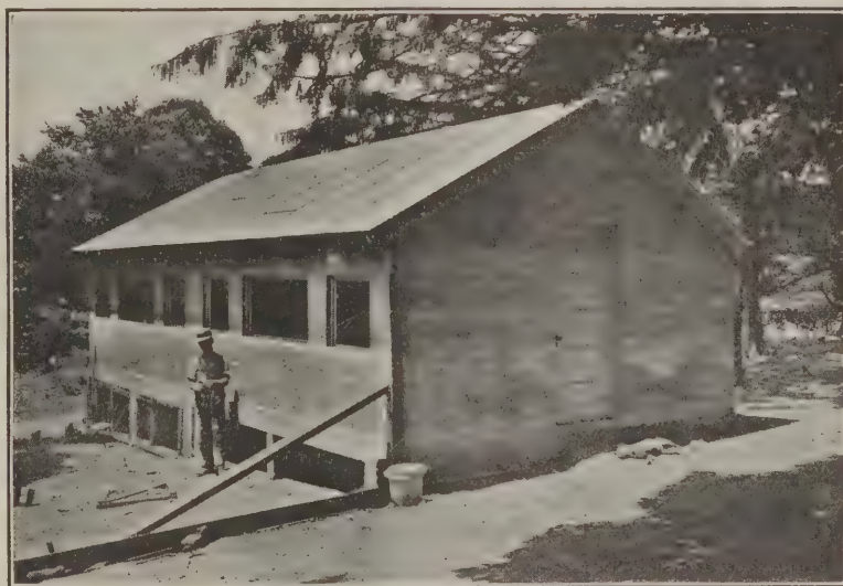
Erecting Small Concrete Buildings. Fig. 1—A Poultry House Resting on Concrete Piers and with Walls 4 In. Thick. Floor and Partition Are Also of Concrete
