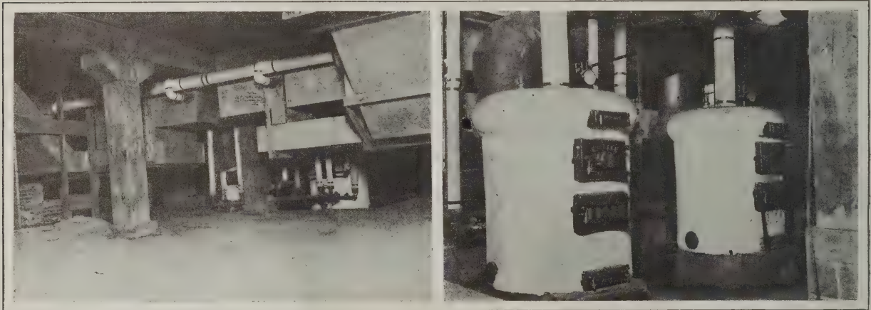
Heating a Two-Story Brick School House—Figs. 6 and 7—Basement Views Showing the Arrangement of the Mains and the General Appearance of the Boilers Used in the Heating Plant
