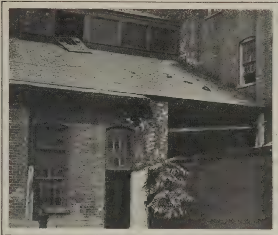
How a Large Truss Roof Was Raised—Fig. 3—A Beam Problem for the Contractor
