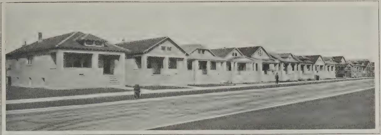
PARTIAL VIEW OF A ROW OF TWENTY-FIVE HOUSES, SOME OF WHICH ARE SHOWN IN PROGRESS OF CONSTRUCTION
