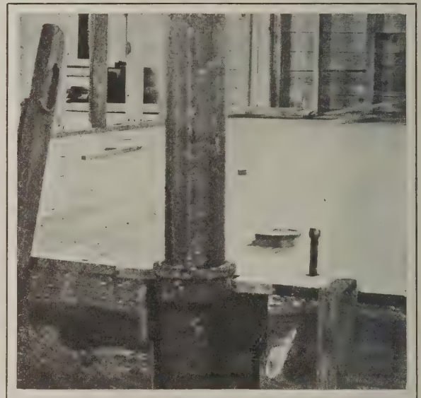
Fig. 10—Showing How Floor Joist Was Mutilated at Second Story Level
