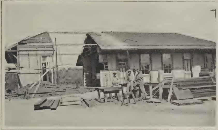
Remodeling a Frame Station Building—Fig. 5—Appearance of the Structure After It Had Been Cut Apart
