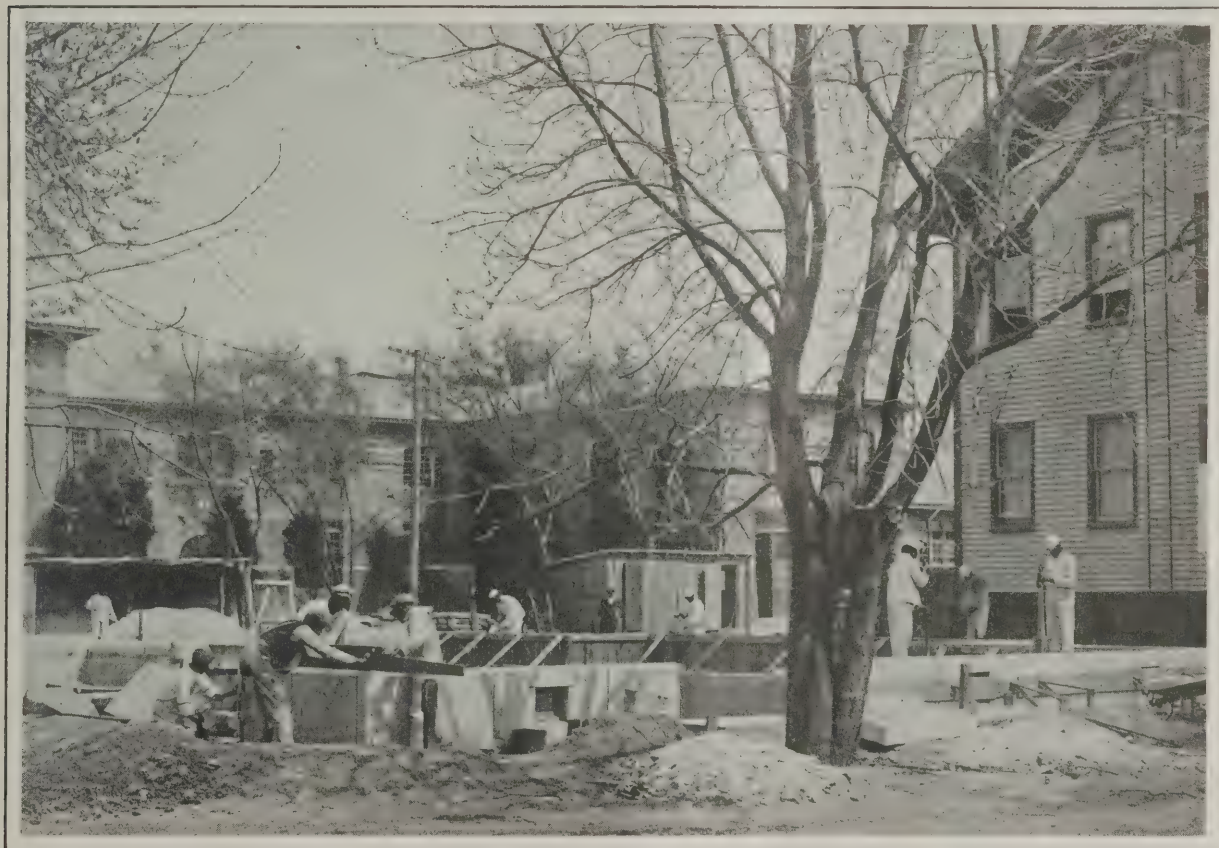
Industrial Education in the South—Fig. 6—Hampton Students Laying the Foundations for the New $30,000 Two-Story Brick Y. M. C. A. Building
