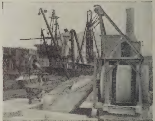
Fig. 12—A "Standard" Low-Charging Concrete Mixer After Four Years' Use
