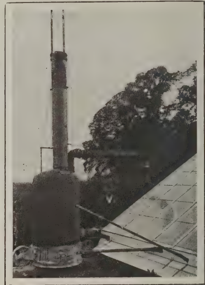
Connections Between Boiler and Portable Greenhouse
