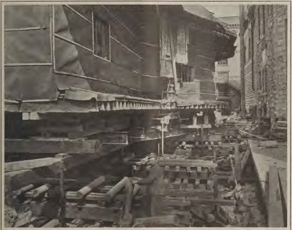
A Notable Church Remodeling Operation—View Showing the Cribbing, Jack Screws, Etc., During the Progress of the Actual Moving of the Building
