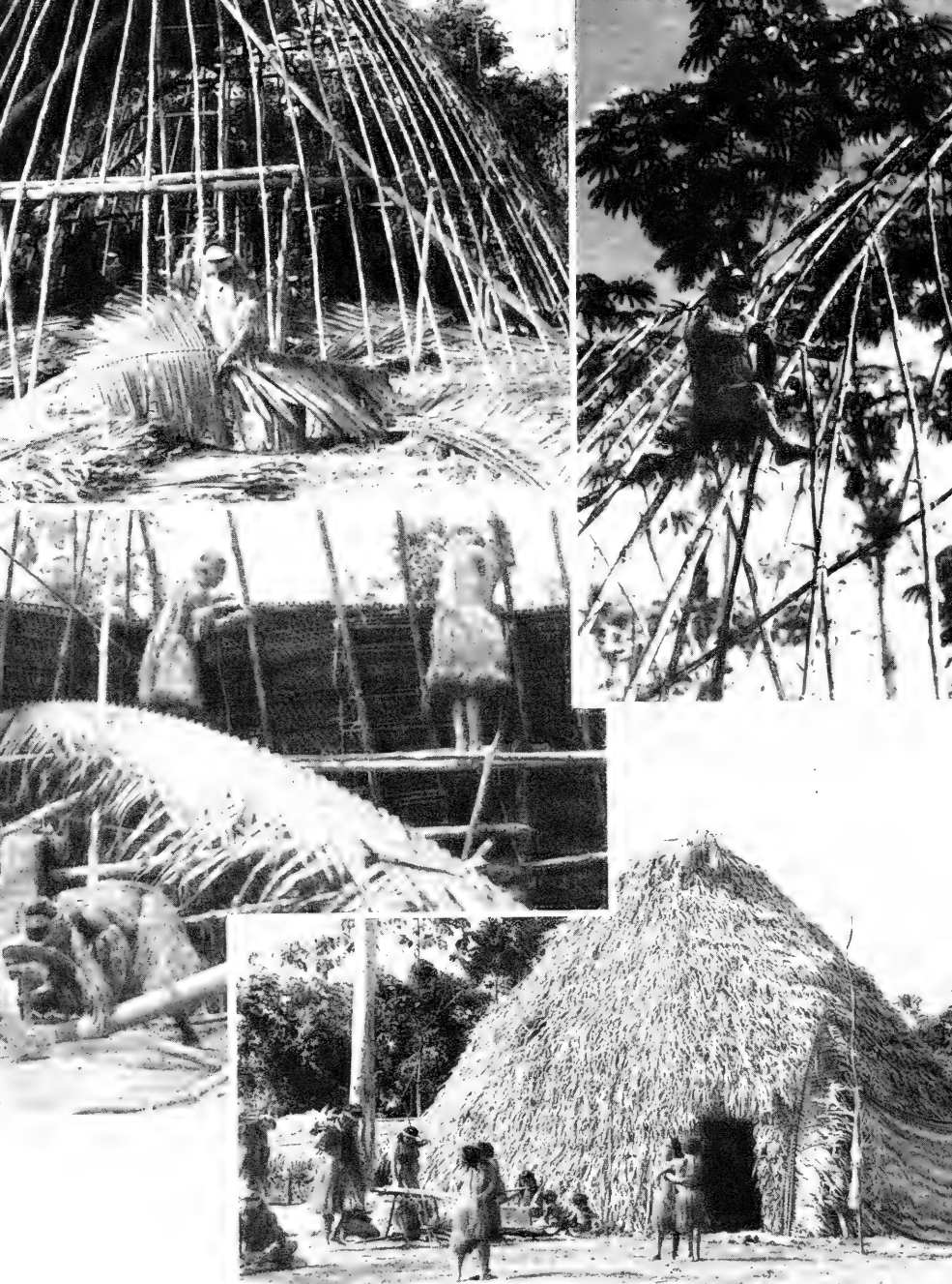
PLATE 69.—Yagua house construction. Top, left: Lower frame arrangement. Top, right: Lashing frame. Bottom, left: Plaiting and placing thatch. Bottom, right: Finished house. (Courtesy Paul Fejos.)
