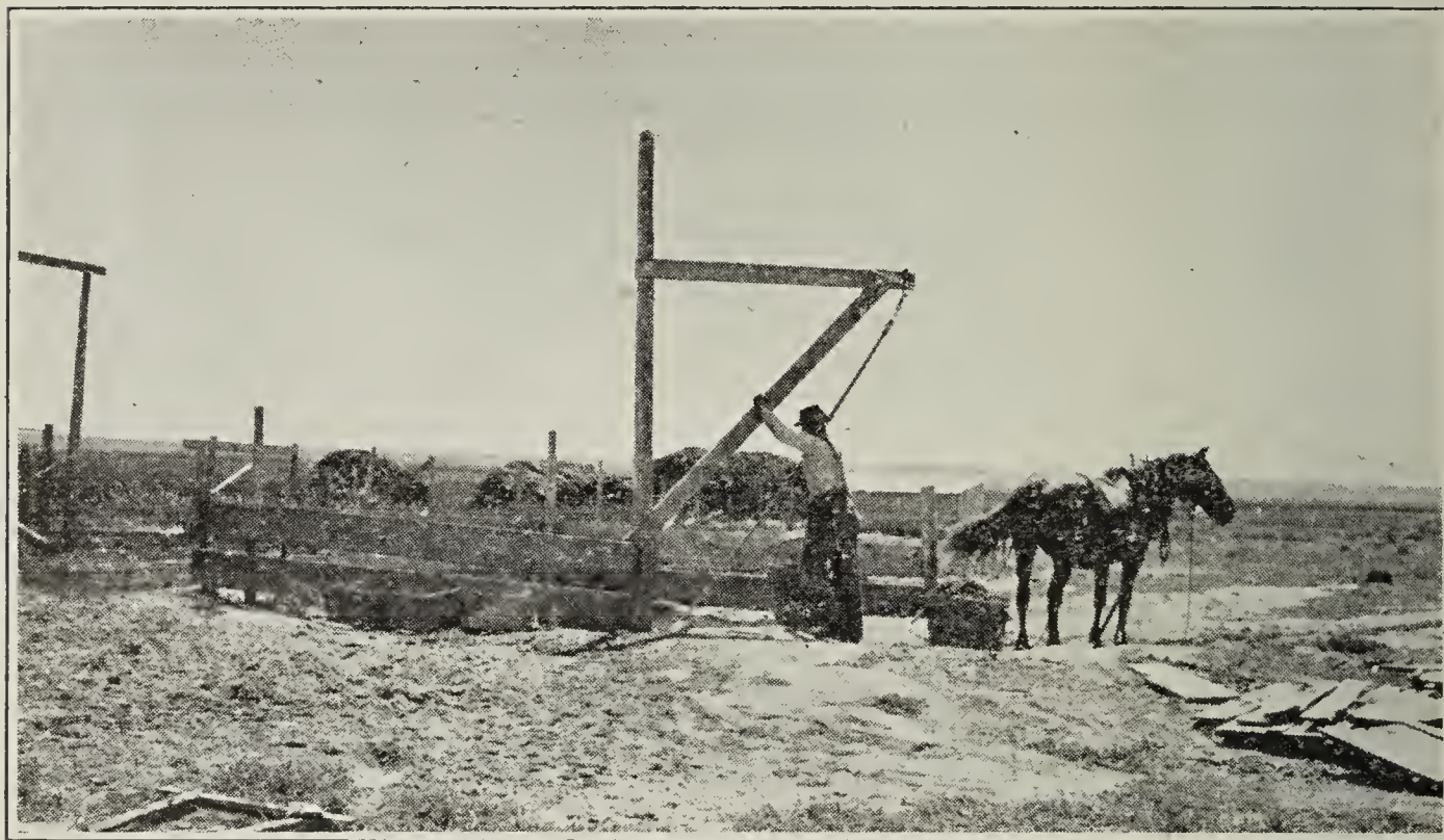
Removing silage from pit silo, the type of silo best adapted to dry-land regions
