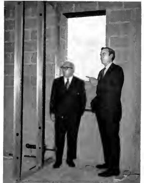
Stanley Armstrong, executive director of the Robert R. McCormick Charitable Trust, and E. Leland Webber, director of Field Museum, look over construction work in a light well area at Field Museum where much-needed additional office and research space is being created for the scientific departments. McCormick Trust contributed $150,000 for the remodeling, in addition to a previous gift of $300,000 for new facilities for the Exhibition Department.
