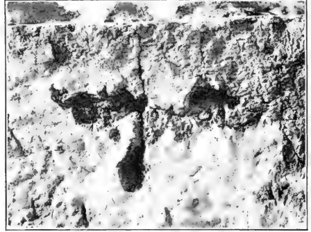
E. Plaster partly removed, showing rectangular checking.
