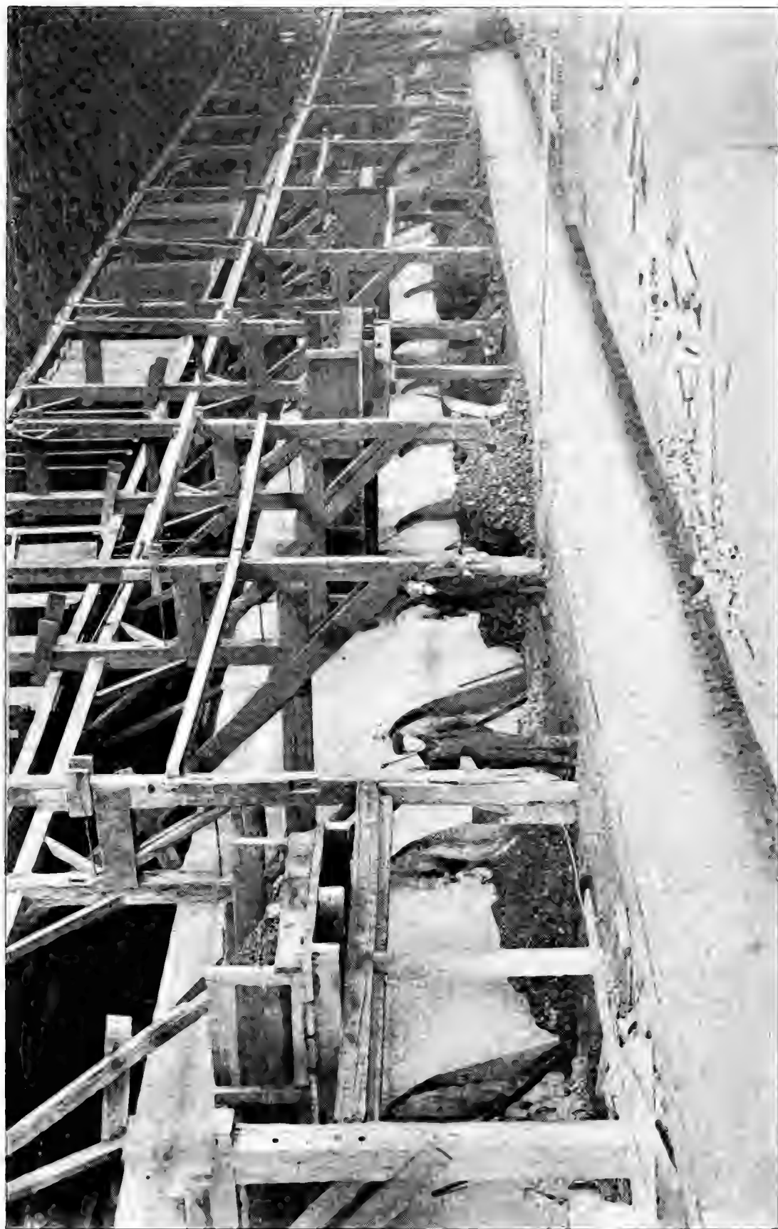
H. Ries photo. Continuous kiln, Haight type, Horseheads brick co., Horseheads. In the foreground is depressed track so that bricks when taken from the kiln can be loaded directly on to the cars.
