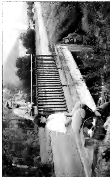
Fig. 7. Terry Hollingsworth and Rchael Thomas by culvert containing communal roost of Old lady moths, 30th July 1994.
