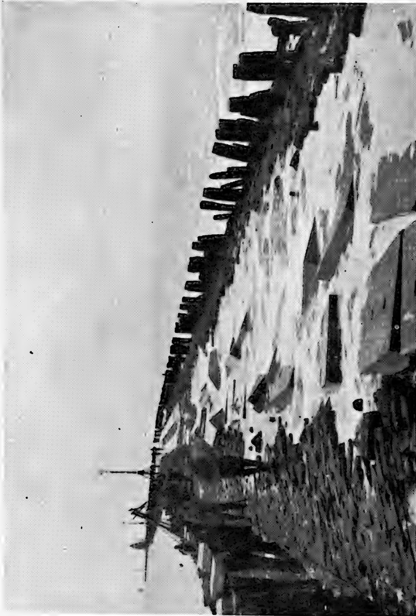
Figure 23. North pier, Hook of Holland. Damage caused by a gale in September 1948 to a section of the track which was completed, but where the asphalt grouting had not been applied. In the background the track is undamaged where provided with asphalt grouting.
