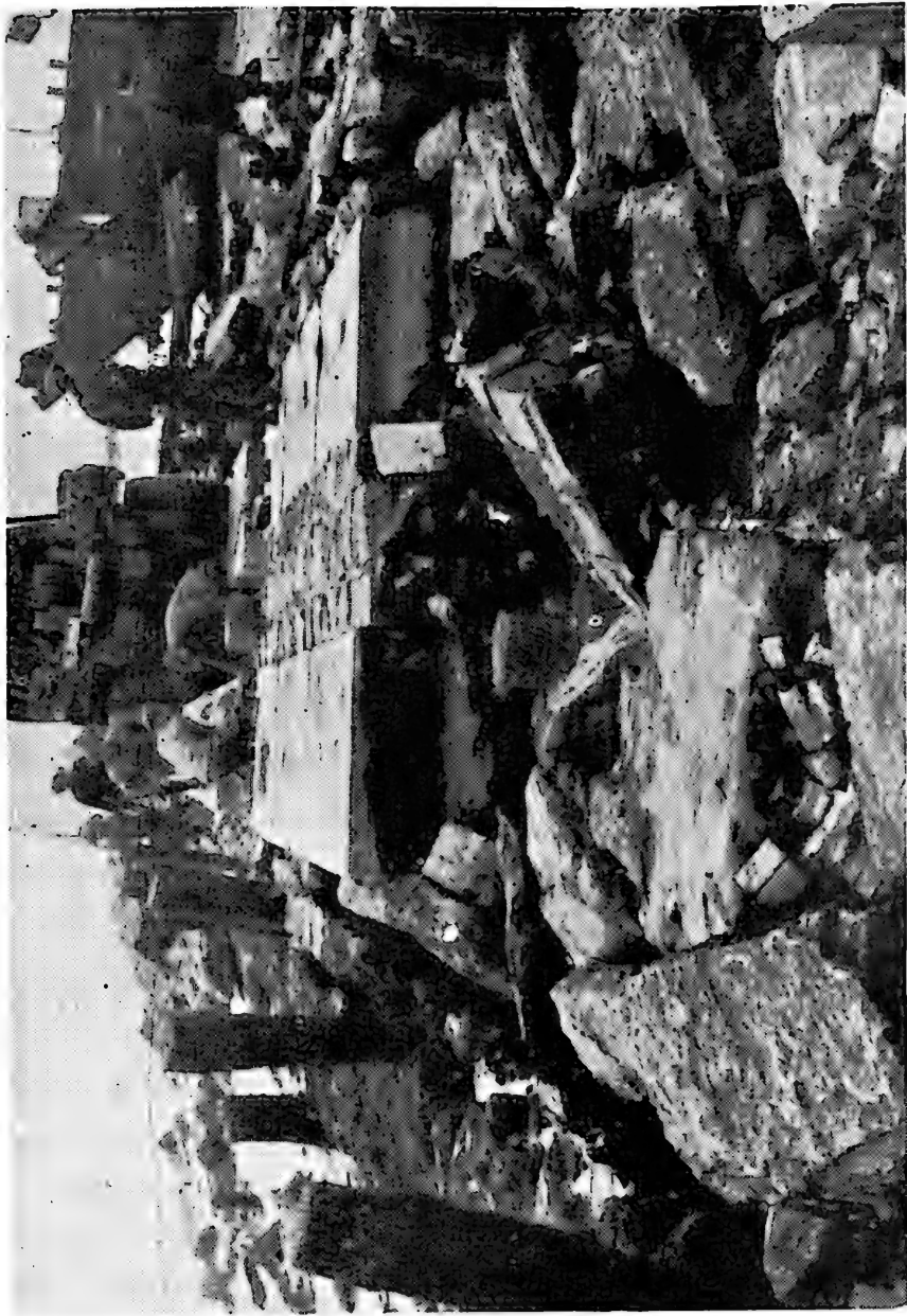
Figure 24. Connecting dam near south pier at Hook of Holland. Damage caused by gale in April 1949 on a short section which was almost completed, but where the sides of the track had not yet been grouted.
