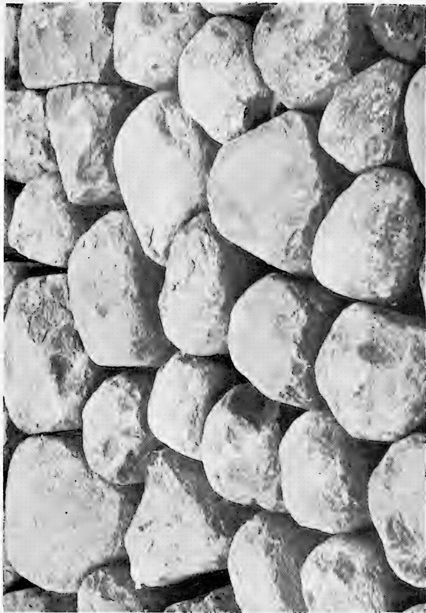
Figure 5. Westkapel sea dike. Riprap of worn basalt before the application of the pouring asphalt.
