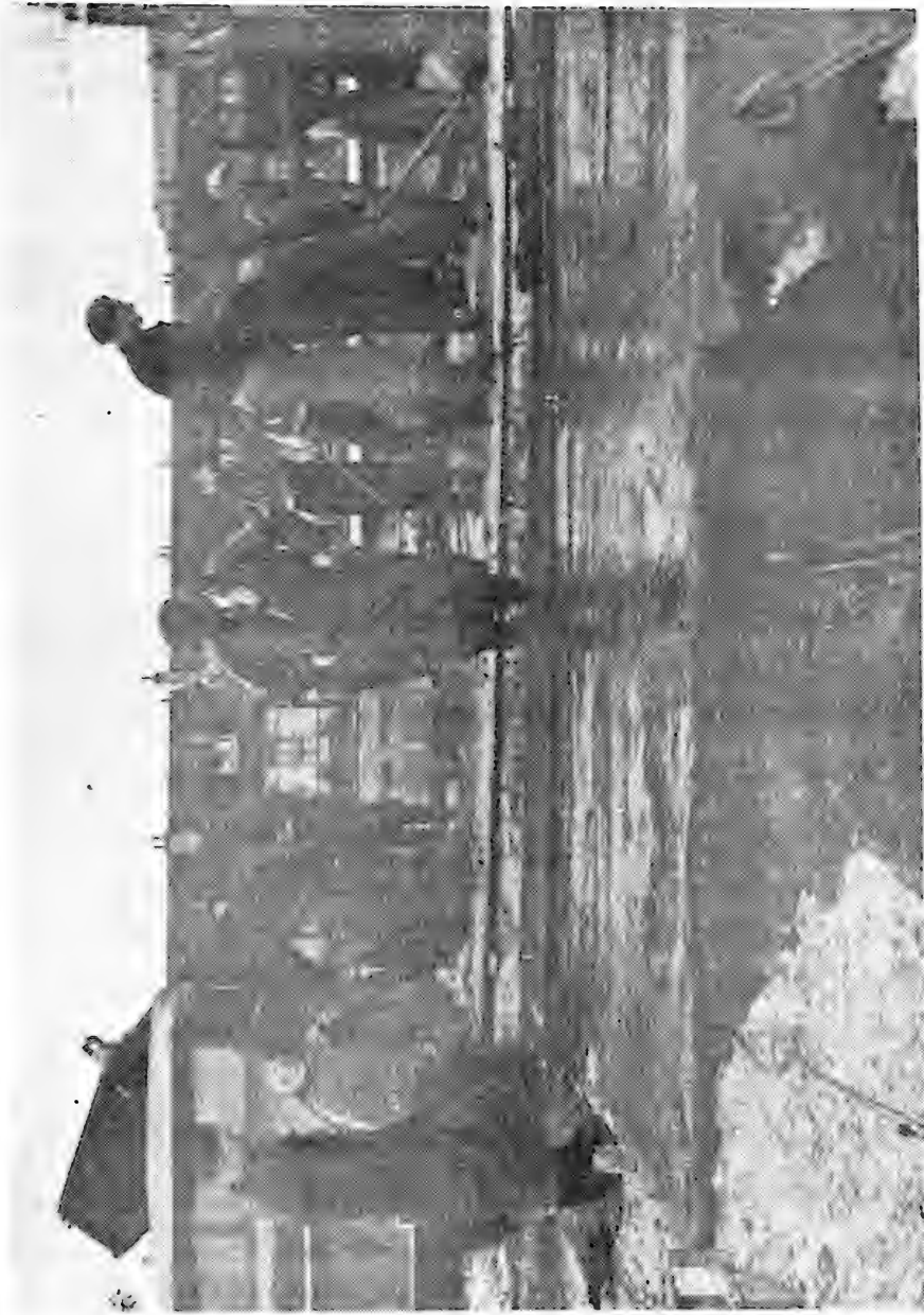
Figure 13. New north harbor at Harlingen. The casting of an asphalt mattress (13 x 5 m; thickness, .15m) being completed on top of first layer (.075 m thick) on which the lifting cables were placed and strung.
