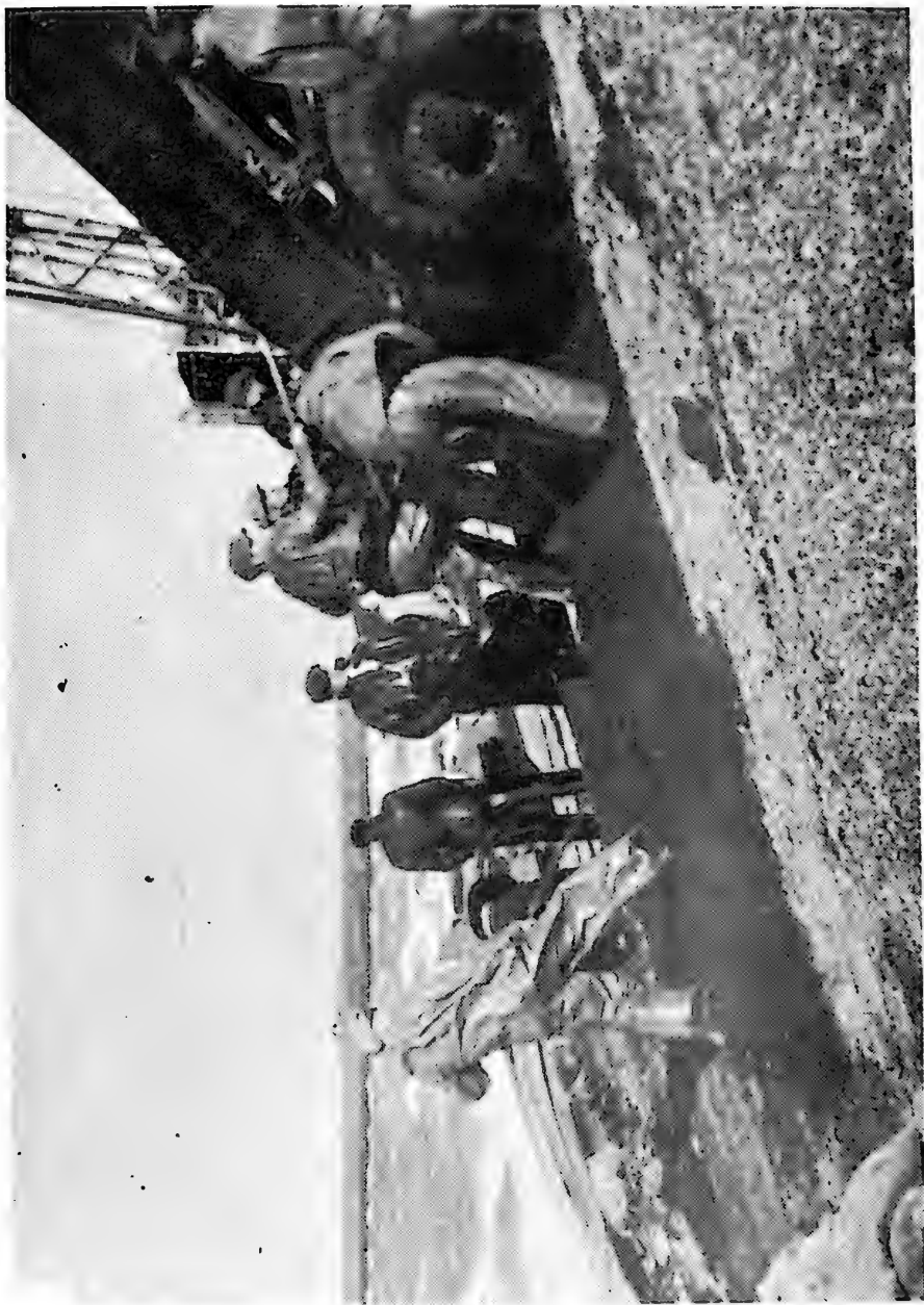
Figure 10. New North harbor dam at Harlingen. Dumping and spreading bituminous sand on the outer slope.
