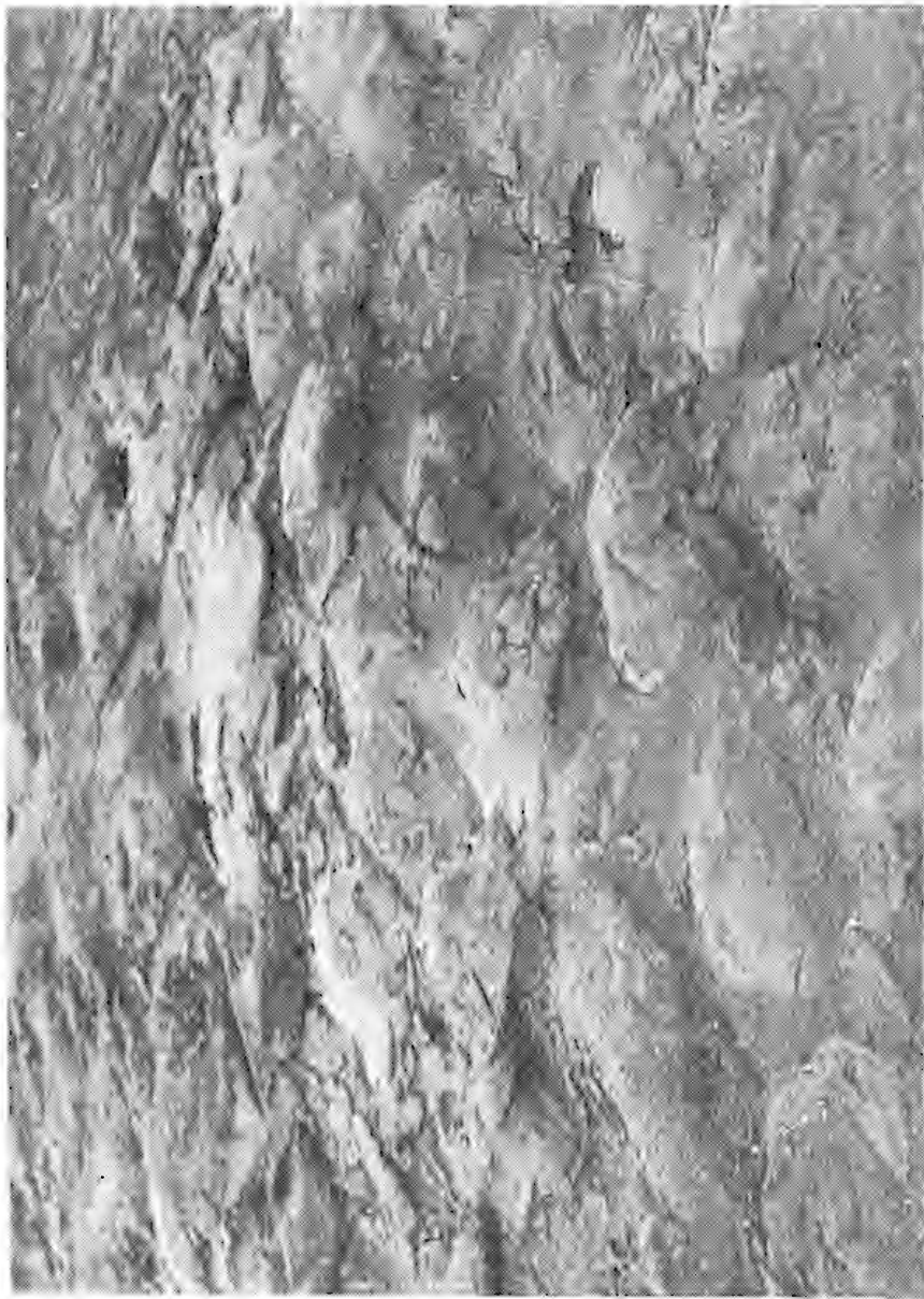
Figure 6. Westkapel sea dike. Westkapel sea dike. Riprap of worn basalt after application.
