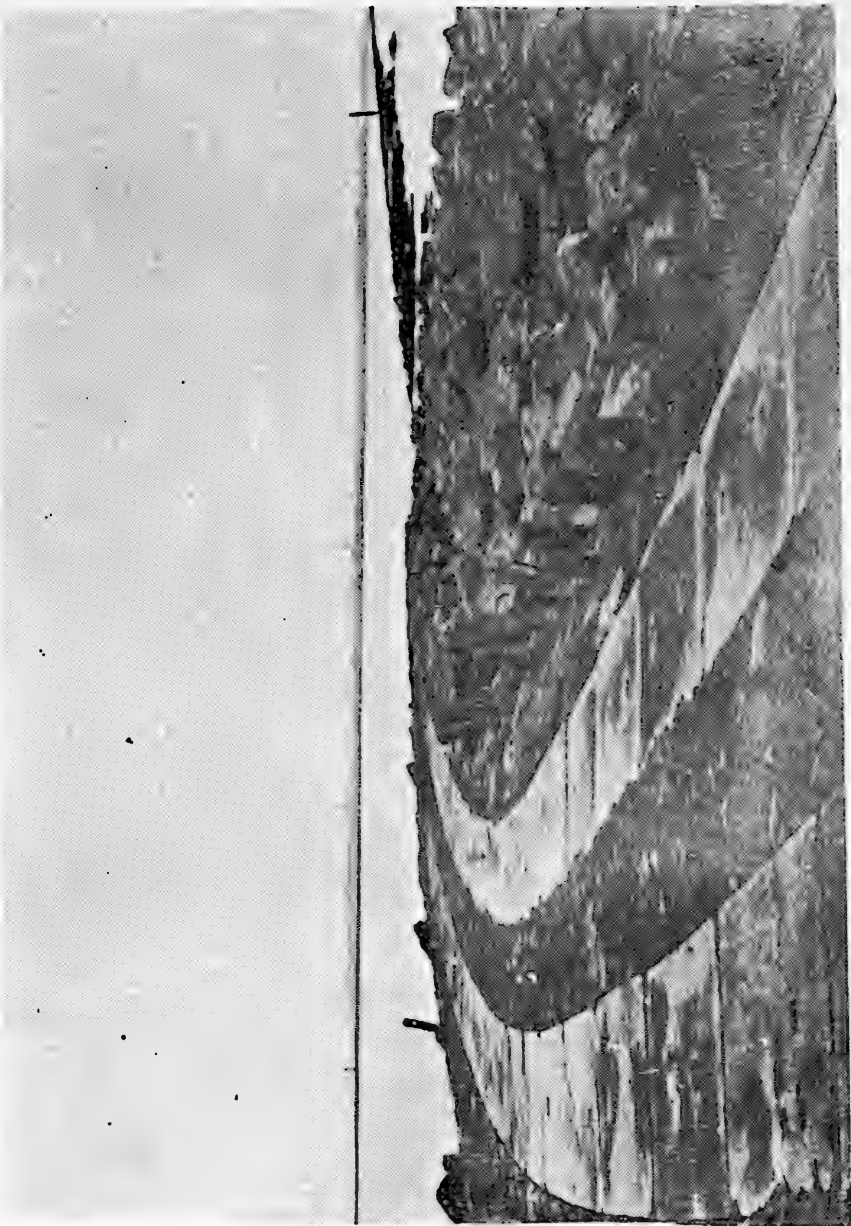
Figure 26. Same view as Figure 25 after reconstruction in winter of 1948-49 and asphalt grouting applied. Picture taken during low water immediately after the heavy gale of 1 March 1949. At the right big boulders from the submarine slope which were carried over the dam by the heavy ground swell.
