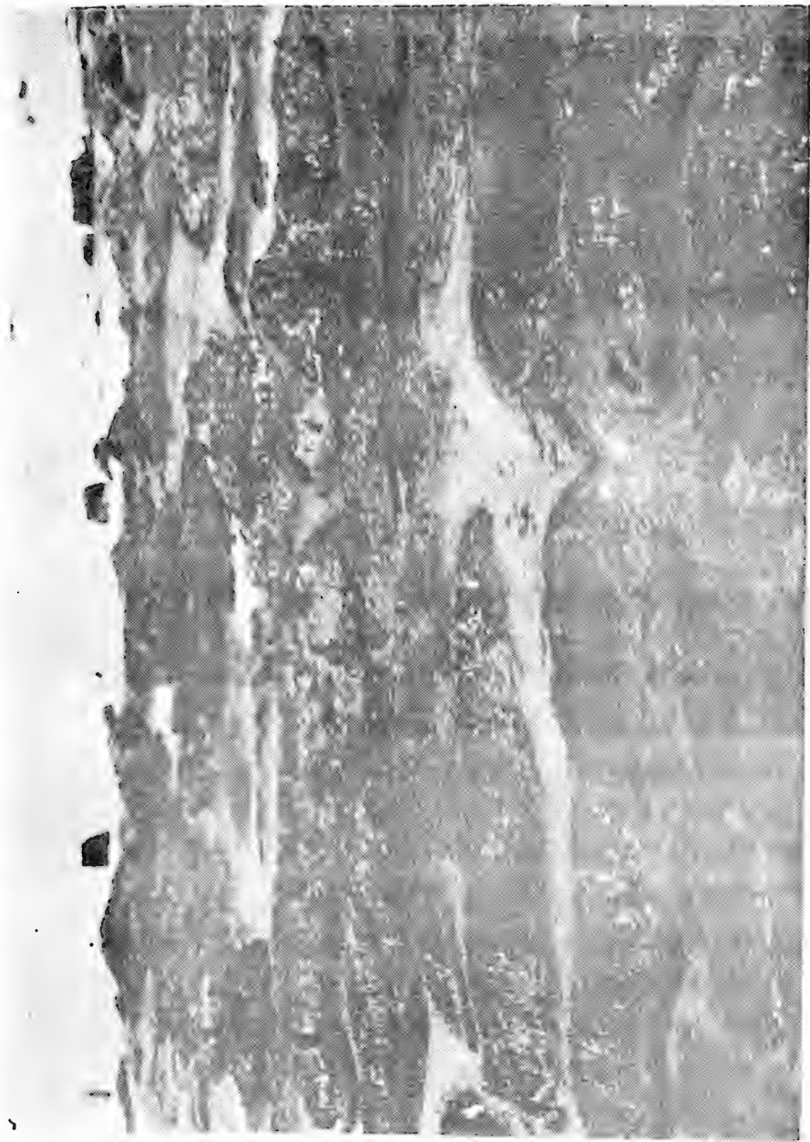
Figure 21. End of the north pier at Hook of Holland. Part of heavily attached stone protection with grouting applied in autumn of 1947.
