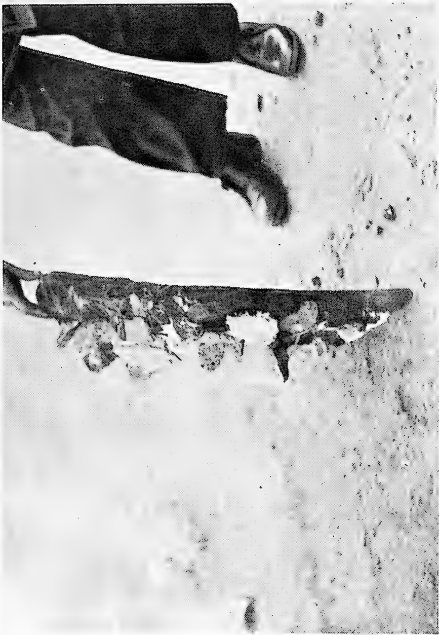
Figure 4. Westkapel sea dike. A fragment torn out of the rubble stone protection penetrated with asphalt mastic.
