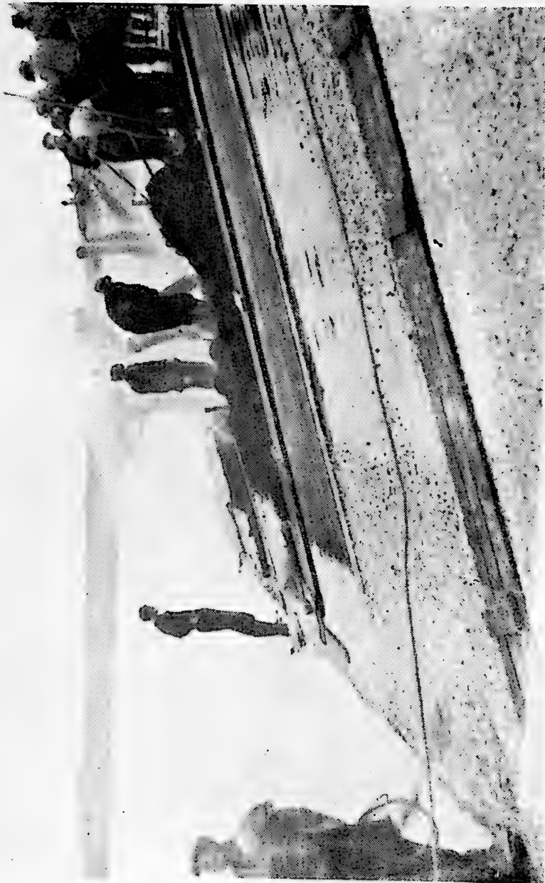
Figure 11. The cover of the outer slope of Harlingen dam being spread, compacted and covered with hot asphaltic bitumen and shells.
