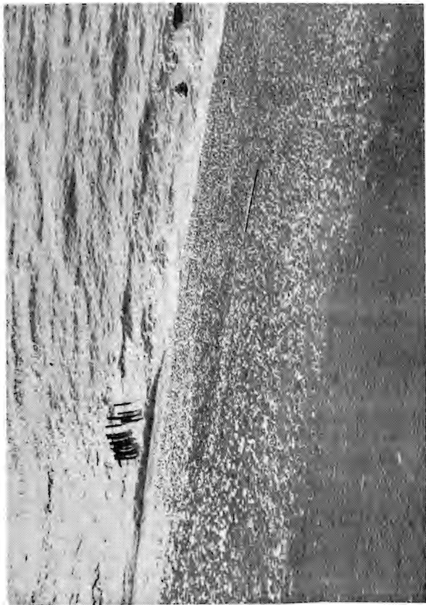
Figure 8. Westkapel sea dike. Slope protection of basalt stone grouted with pouring asphalt.
