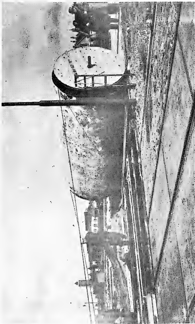
Figure 17. An asphalt mattress, 15 x 5 m, .06 m thick, weighing 9 tons, being wrapped around a drum. (Harlingen).
