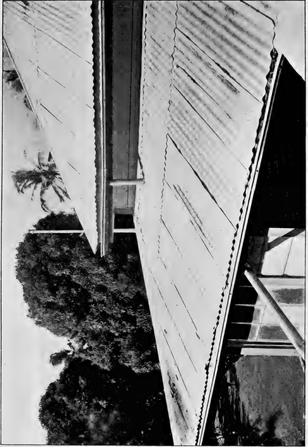
Sagging eave-troughs in which larvæ and pupæ of Stegomyia fasciata were abundant.
