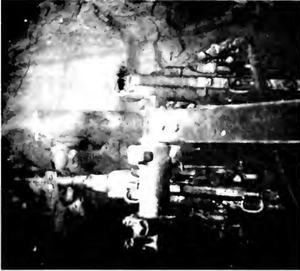
Figure 6. HOOSAC TUNNEL. Flash-powder photograph of Burleigh drills at the working face. (Photo courtesy of State Library, Commonwealth of Massachusetts.)
