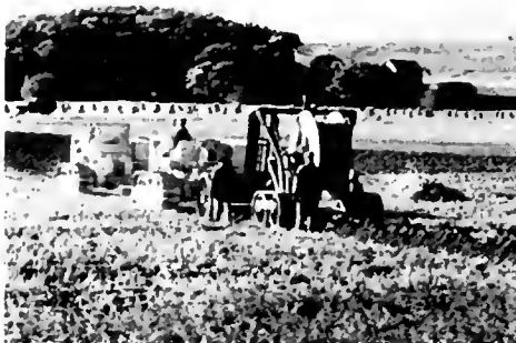
PLOWING IN COAXIAL CABLE ON THE LONG ROAD from Stevens Point to Minneapolis is shown in this typical scene from "Coaxial," an industrial saga of the telephone business.
