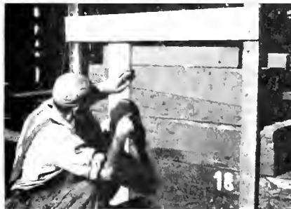
A shifting line scribed into wood serves as tell-tale should blocks shift out of position
