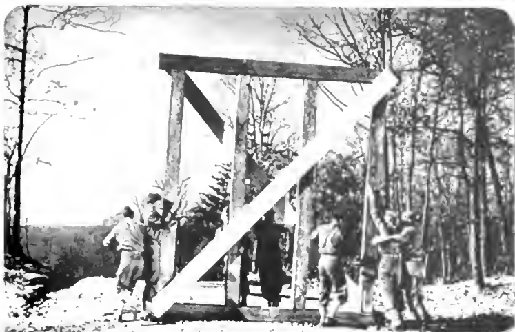
1. Soldiers build small trestle to be carried to its position at the bridge site.
