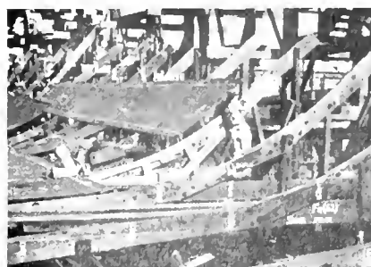
After spauls are in position, final checkup is made with template mold
