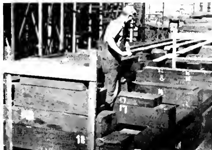
A chalkline pulled tight over the straight edges is at correct declivity angle
