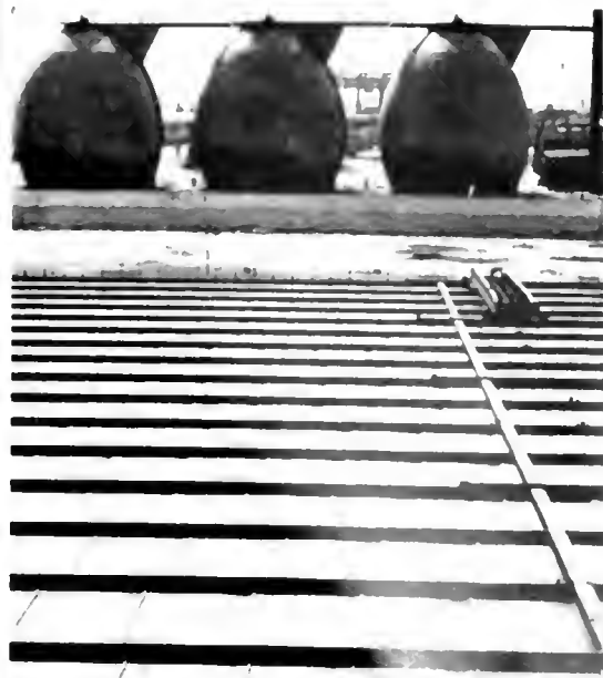
Modern sewage treatment work is pictured in "The River Must Live" as a part of the answer to the elimination of pollution.
