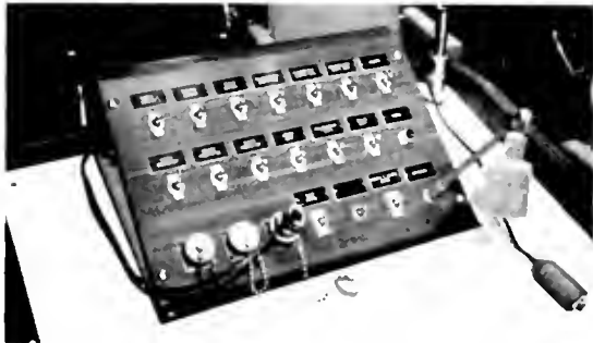
The control panel is mounted on the lectern but may be easily removed and used anywhere in the room; a twin panel is in the projection area. Screens, projectors, recorders, players, lighting effects and drapes can all be operated by the man in booth or speaker in the meeting room.
