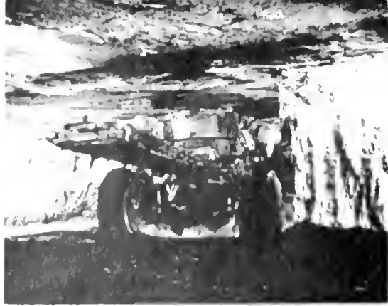
Cutting machine with a nine-foot blade like a giant chain saw moves into coal seam face in Franklin No. 25 mine at New Athens, Ohio. Machine cuts six-inch slot along the base of seam.
