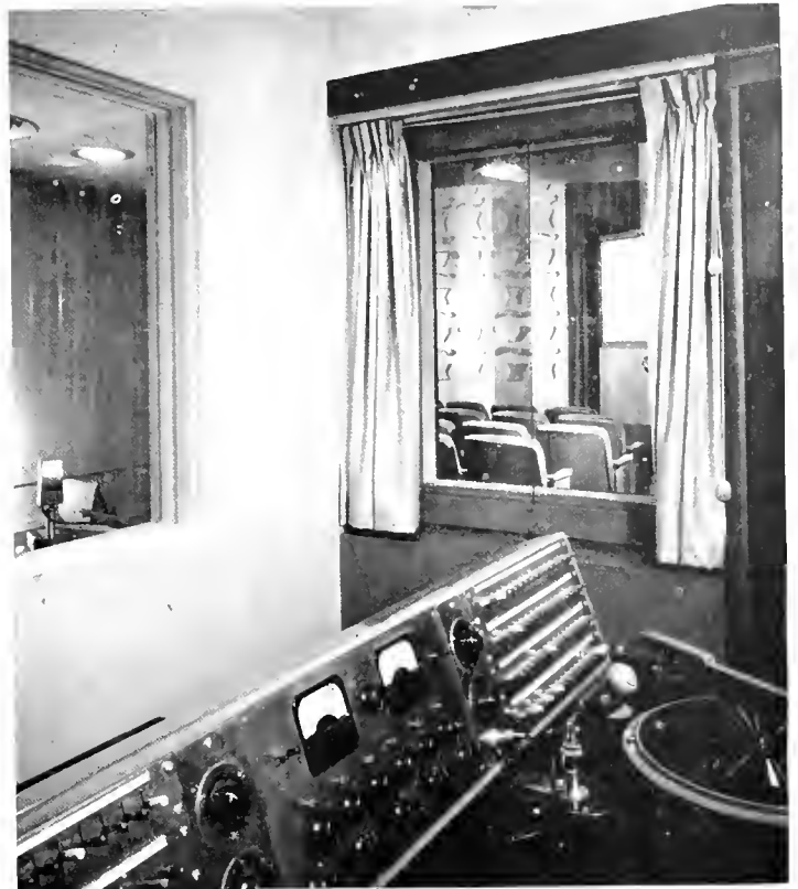
From the vantage point of this sound control room, the "announce" room (left) and theatre can be viewed through sound-proof glass.
