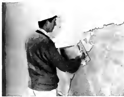
PLASTERING SKILLS are illustrated in the 161 slidefilm from the series "Careers in the Building Trades" (An vocational guidance.)
