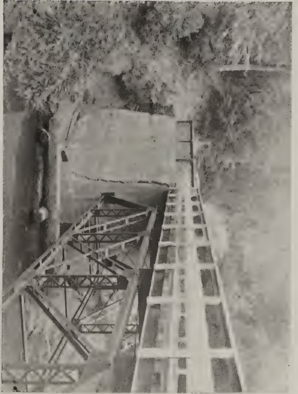
A. Near Watsonville. Concrete pier of bridge shattered. Per J. C. E.
