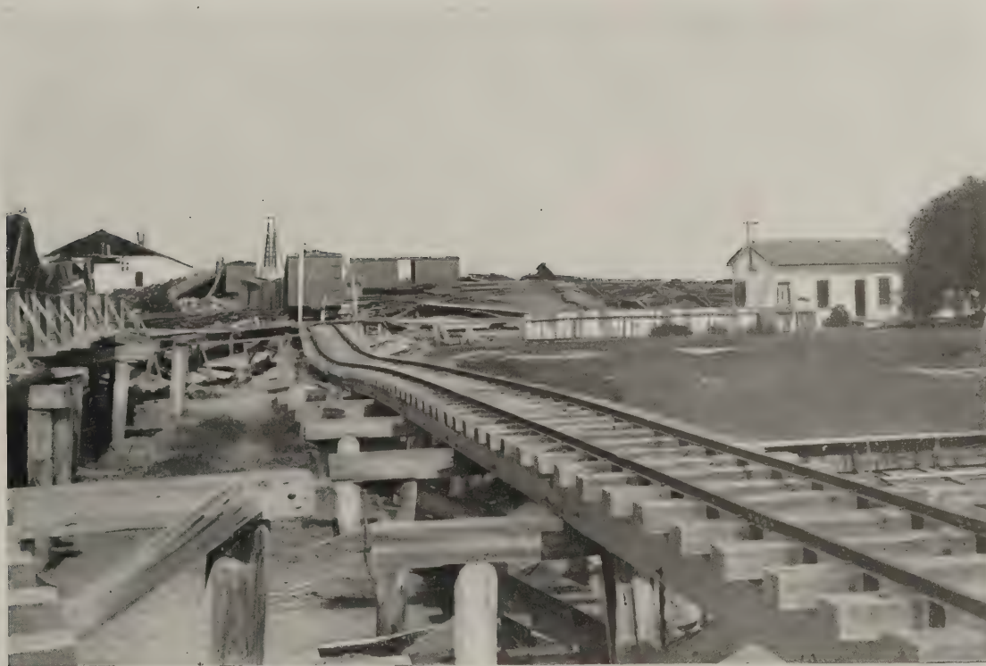
B. Moss Landing. Lurching of ground toward Salinas River carried piles from beneath bridge timbers, causing it to collapse. A. C. L.
