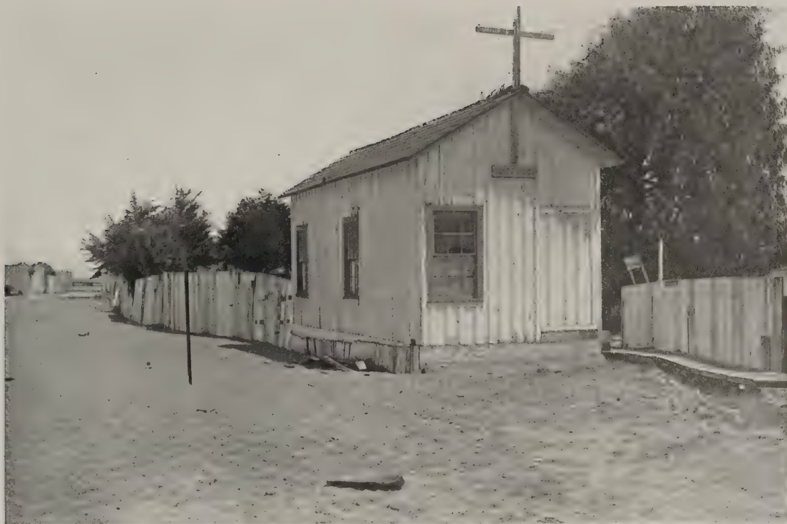
A. Moss Landing. House, tree, and fence moved 12 feet by lurching of ground toward Salinas River. A. C. L.
