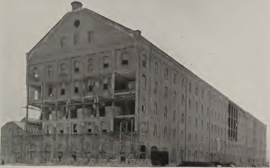
A. Spreckels sugar mill, near Salinas. Entire building buckled. Looking southeast. R. L. H.
