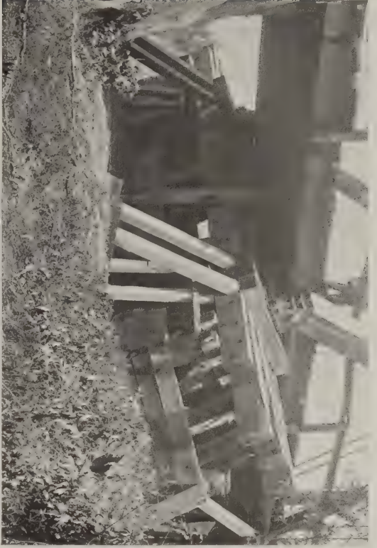
A. Bridge over Salinas River, 4 miles south of Salinas. South terminal pier thrust south 7 feet. A. C. L.
