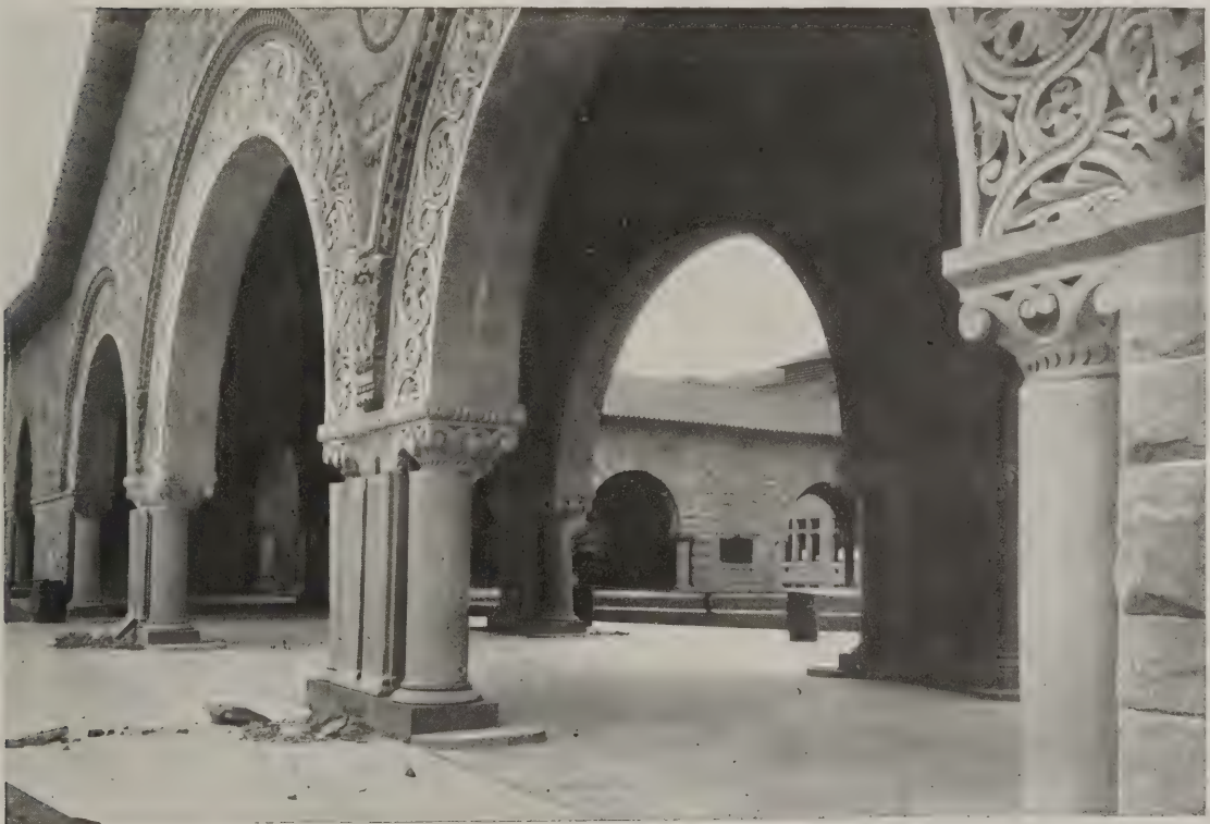
B. Arches that moved on their supporting columns, Stanford University. Per J. C. B.
