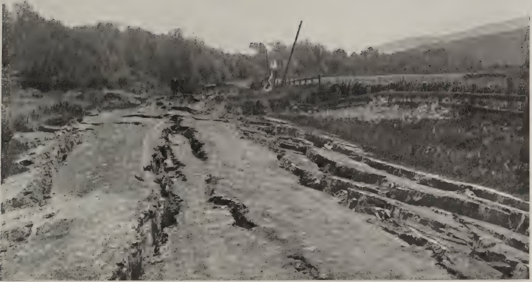
A. Lurching of ground toward Salinas River and consequent collapse. Near Spreckels. A. C. L.
