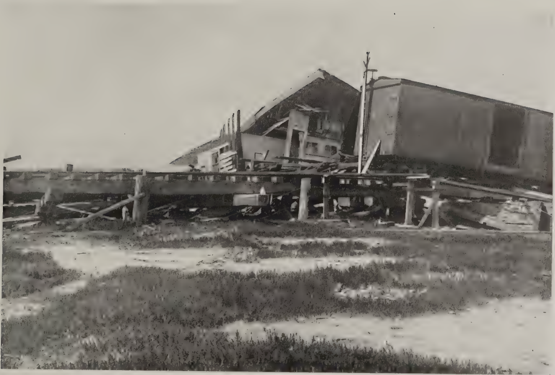
A. Moss Landing. Lurching of ground toward Salinas River, to left, carried piles from beneath bridge timbers and caused bridge to collapse. Displacement 9 feet. A. C. L.
