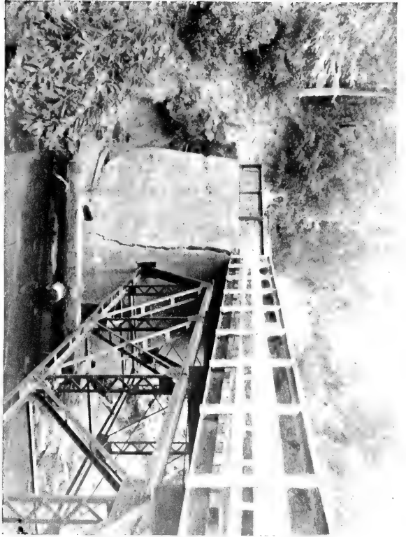
A. Near Watsonville. Concrete pier of bridge shattered. Per J. C. B.
