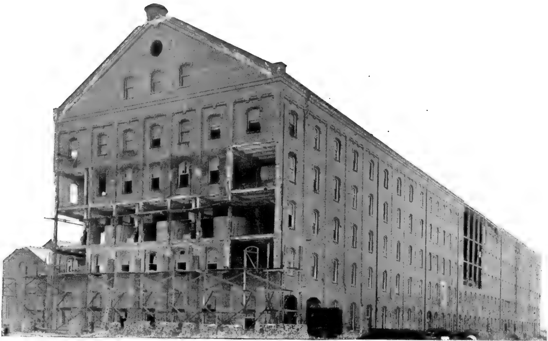
A. Spreckels sugar mill, near Salinas. Entire building buckled. Looking southeast. R. L. H.
