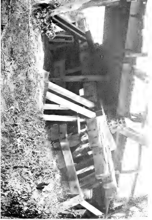
A. Bridge over Salinas River, 4 miles south of Salinas. South terminal pier thrust south 7 feet. A. C. L.
