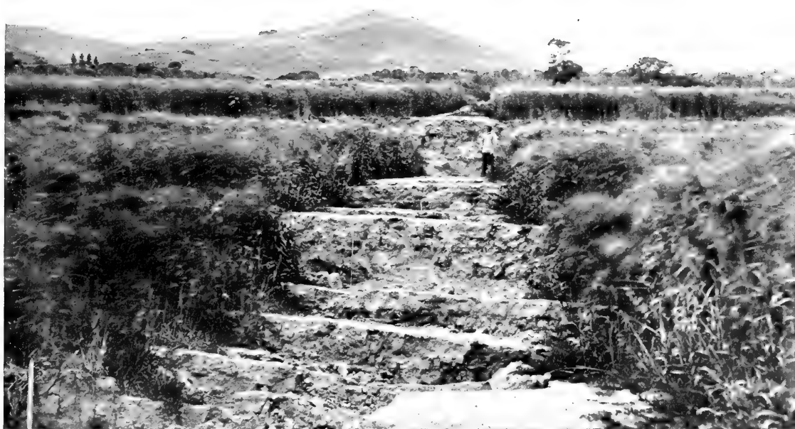
A. Lurching of ground toward Salinas River, with consequent collapse. Near Spreckels. Per J. C. B.
