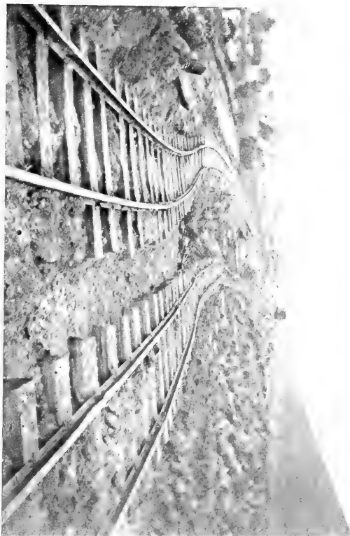
A. Earth-slip north of Tomales, carrying railway roadbed with it. Track was straight before earthquake. R. S. H.
