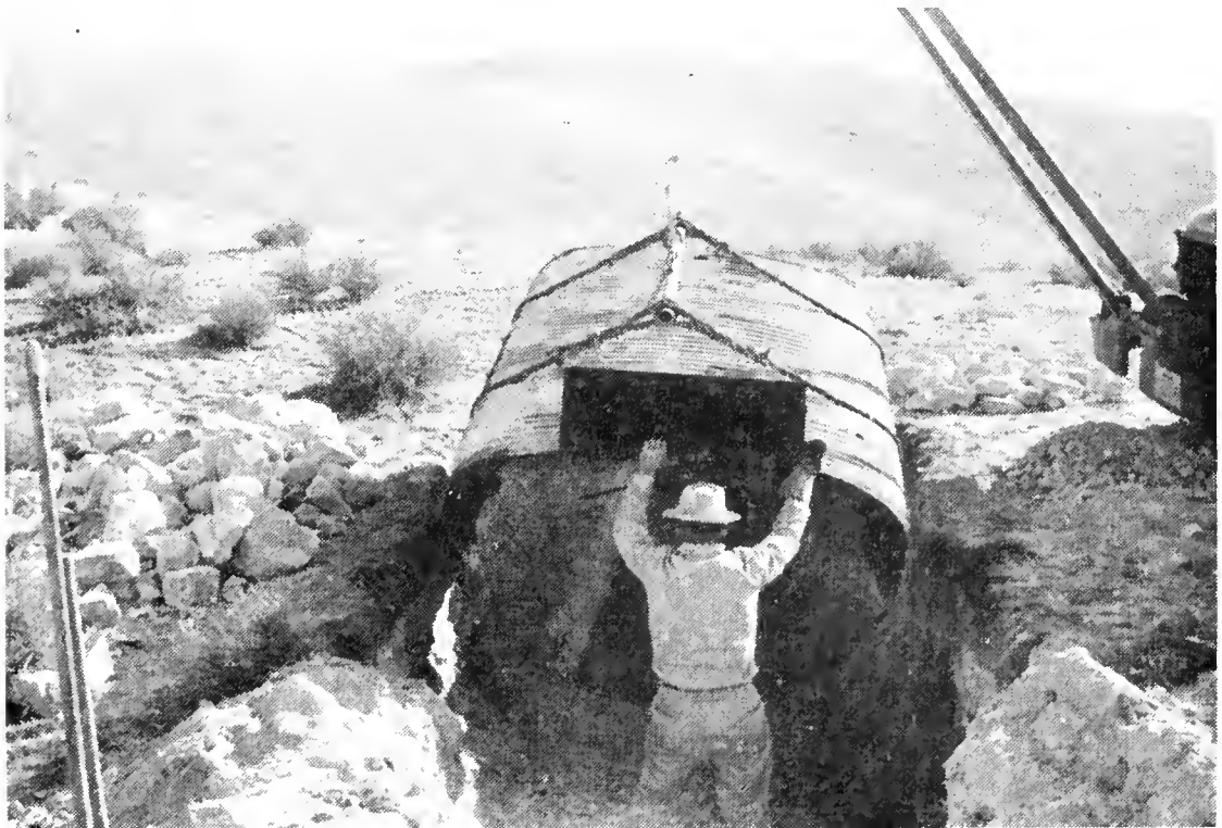
FIGURE 12. A 1,200-gallon steel guzzler in the process of being installed in the Temblor area. The main part of the tank is asphalt-dipped, asbestos-bonded, corrugated arch pipe. The end plates are asphalt-dipped galvanized metal. Photograph by H. Harper.
