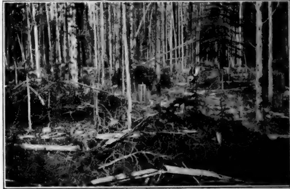
Slash on logged over area piled so as to reduce fire danger. All the contractors working on the 2,000 miles of railroad being constructed in B.C. are now required to pile slash.
