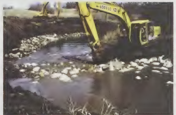
Figure 18.3. Creation of a riffle on Cox Creek, Cass County. Riffle construction involves the use of heavy equipment and causes temporary disturbance of the site. Photo by J. Rodsater.
