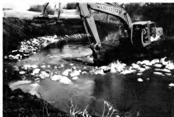
Figure 18.3. Creation of a riffle on Cox Creek, Cass County. Riffle construction involves the use of heavy equipment and causes temporary disturbance of the site. Photo by J. Rodsater.
