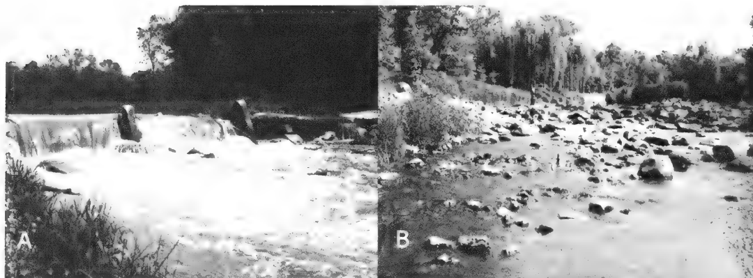
Figure 18.4. Removal of a dam on Waubensee Creek in Kendall County. Replacement of the dam with a constructed riffle allows fish passage. A) before, B) after. Photos by J. Rodsater.
