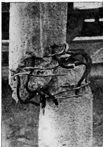
FIG. 77.—Overloaded Column, with Insufficient Longitudinal Reinforcement.
