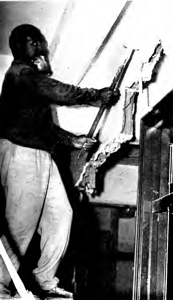
A workman continues banging at the plaster and knocking down a wall to transform the old administration building.
