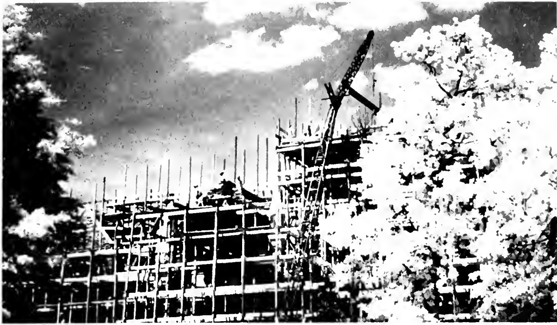
This fall we returned to find that, as seen through the scaffolding, the new administration building was nearing completion except for the many inside details.
