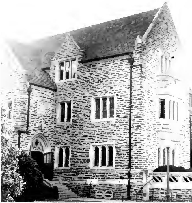
The swift-moving men on the wrecking and rebuilding crews are aiding the old administration building to become a modern student center.
