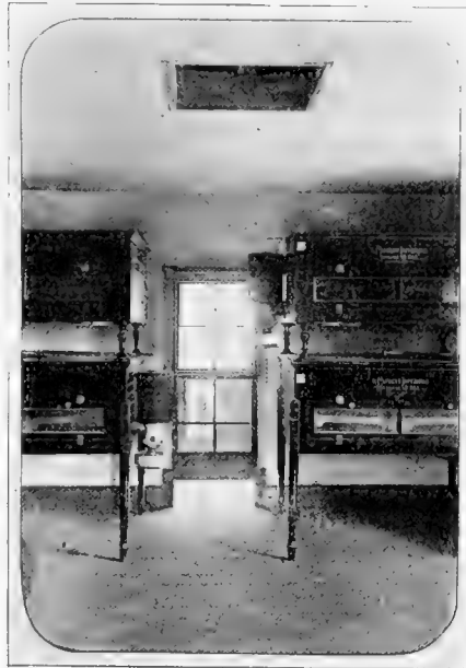
Ventilating Openings in Ceiling and Window in Incubator Room on Jordan Poultry Plant.
