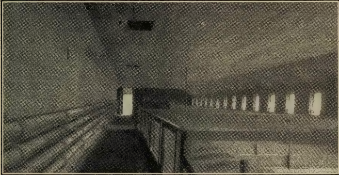
Interior of a Brooding House, Showing the Pipes Which Heat the Hovers and Also the Four-Inch Cast Iron Pipes Which Warm the House.
