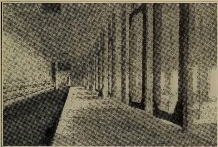
Interior of a Brooding House Equipped With What is Known as a "Box" Hover. This Hover is Open Only at the Front, Into the Pens, and is Heated by Hot Water Pipes.
