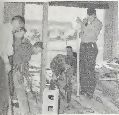
Mr. Jesse Grimes, advisor, super- vises boys working on the Fire Department Building.
