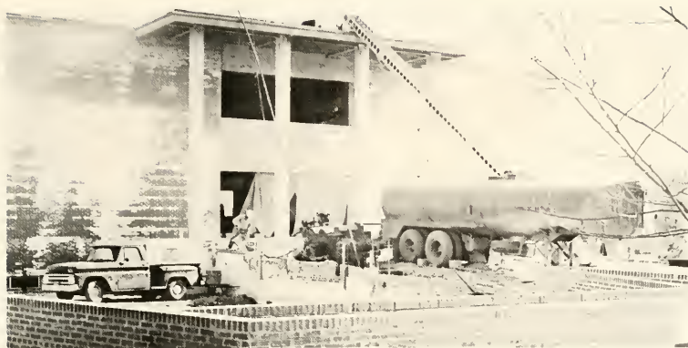
The Whitaker Library and Fine Arts Building is expected to be completed and ready for use by the beginning of the fall term.
