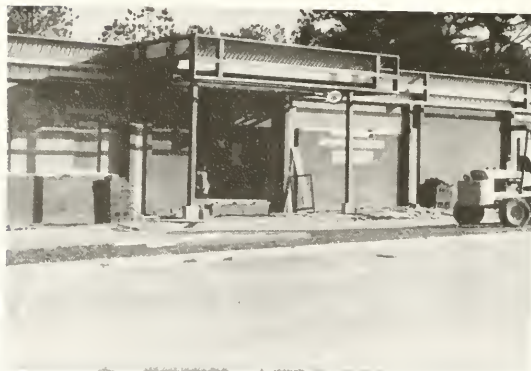
The new Graphic Communications building, to be occupied in the summer of '83
