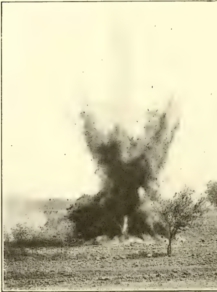
FIG. 46. — Breaking a layer of hardpan by means of a stick of dynamite discharged in each tree hole.
