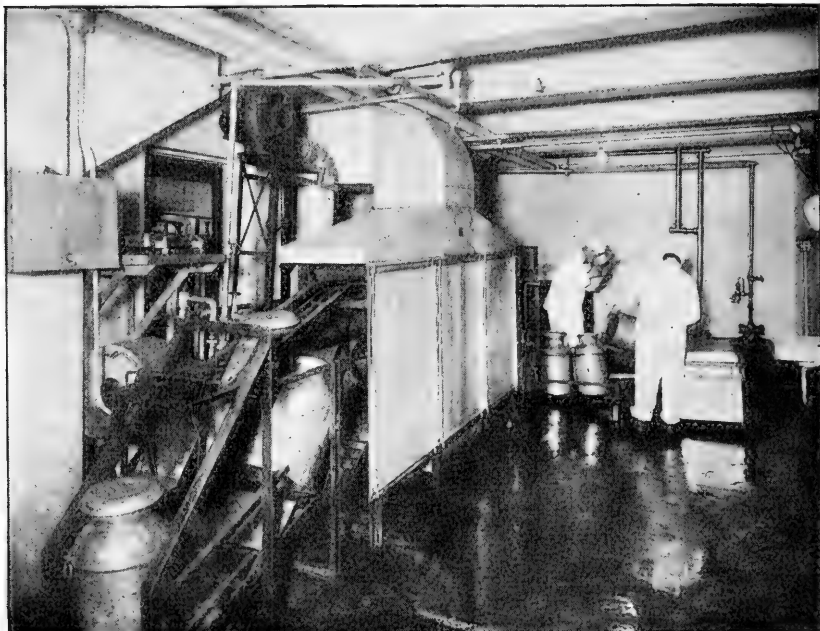
FIG. 7.—Receiving room with can washer.
