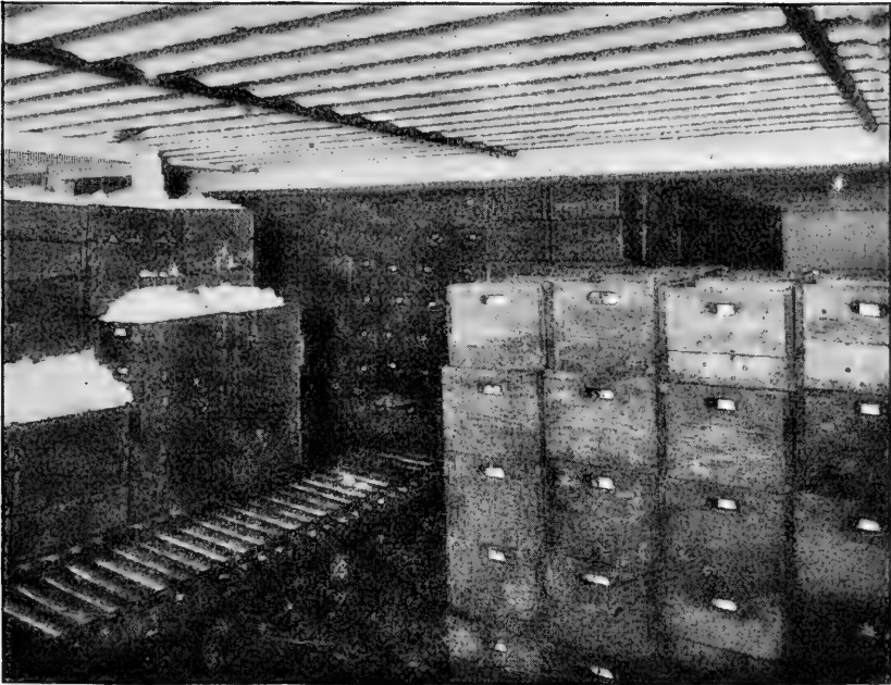
FIG. 10.—Milk-storage room using direct system of cooling with cooling coils overhead. Note iron plates in floor.
