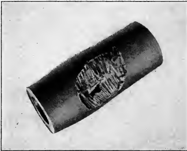
FIG. 85. Lead pipe gnawed by rats
