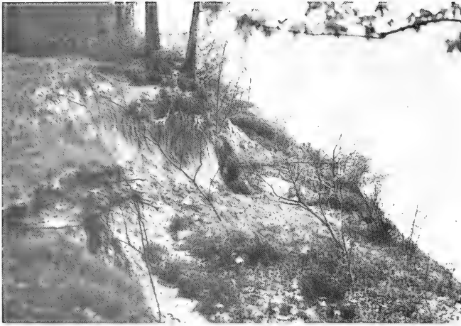
8 May 1973 - Large-scale slump of upper part of till bluff.
