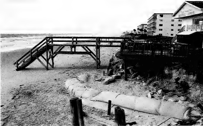
Figure D-21: Noro and Co. property, May 9, 1996, showing the deteriorated wooden bulkhead and geotextile sandbags, as well as storm-induced erosion to the dune face (source: N. C. Kraus).
