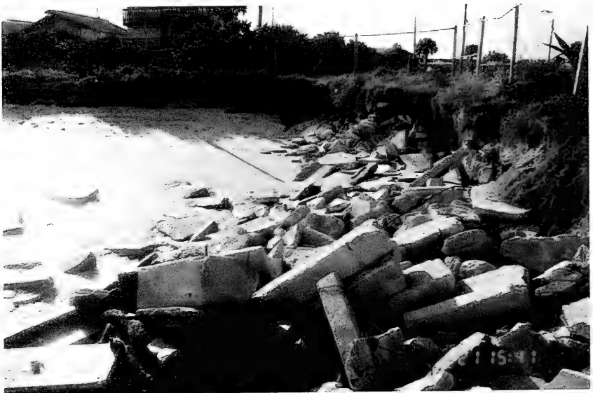
Figure D-15: Southern property boundary of Applegate residence, November 21, 1996, showing downdrift impacts of rubble mound seaward of the structure (source: N. C. Kraus).
