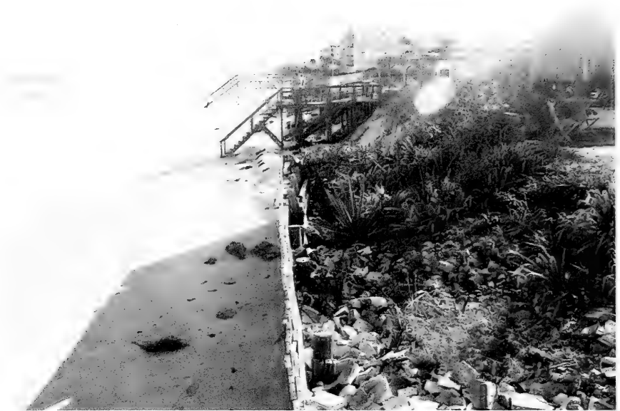
Figure D-26: View south towards Noro property showing the eroded dunes on one property and the creative armoring structures on the neighboring property to the north (source: N. C. Kraus).
