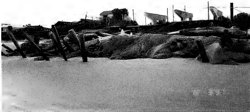
Figure 4-3. Seaward side of the Applegate property, December 3, 1997. Main structure was removed by Mr. Applegate around September 1997; however, the foundation of the dwelling and the rubble in front of the structure still remained (source: N. C. Kraus).
