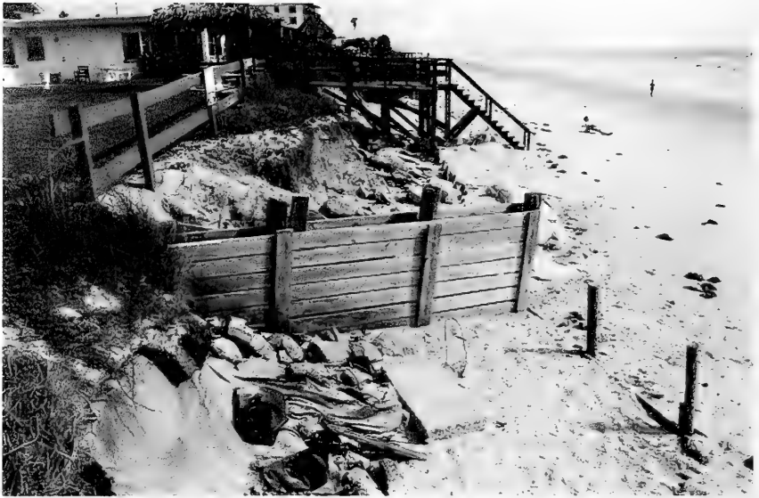
Figure D-22: View north from Noro and Co. property, May 9, 1996, showing storm damage to the dunes and the remains of attempts to protect upland properties (source: N. C. Kraus).
