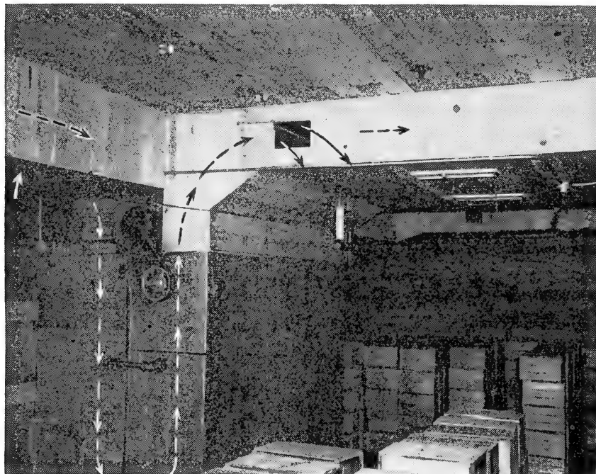
FIGURE 7.—Unit cooler installed with air ducts to deliver the cold air throughout the room and to pick up the return air from the warmest parts, in contrast with the installation in figure 6, where the return air comes from the floor.
