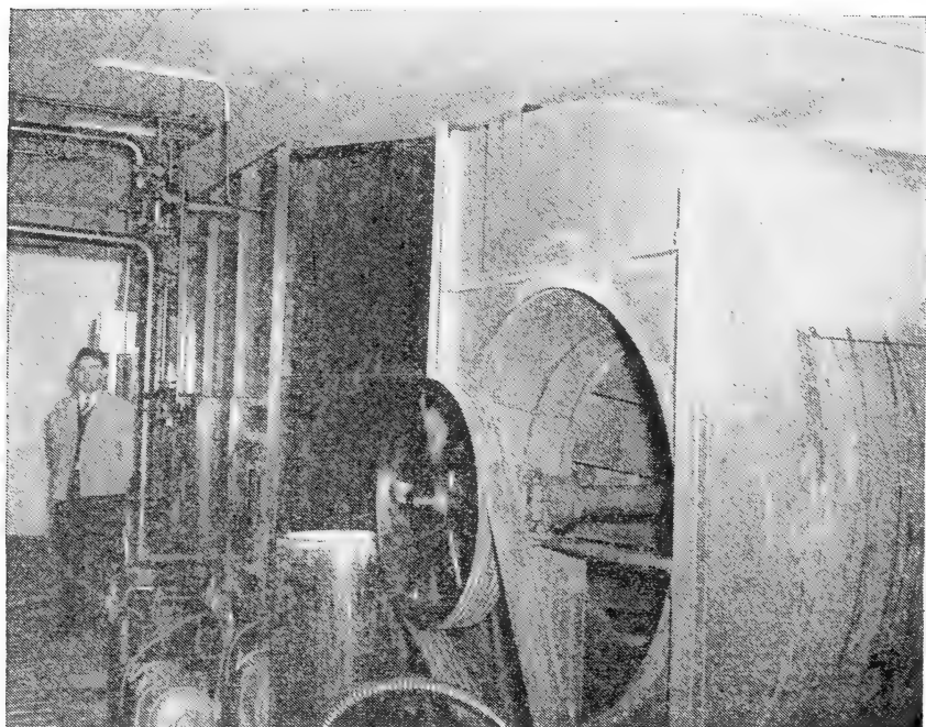
FIGURE 5.—Arrangement of blower and enclosed brine-spray compartment in a brine-spray system. Motor and brine pump for forcing the brine spray over the enclosed evaporating coils are shown at left foreground. In this plant the return air ducts end in the room containing this equipment. The cold-air delivery ducts extend from the farther end of the brine-spray compartment.
