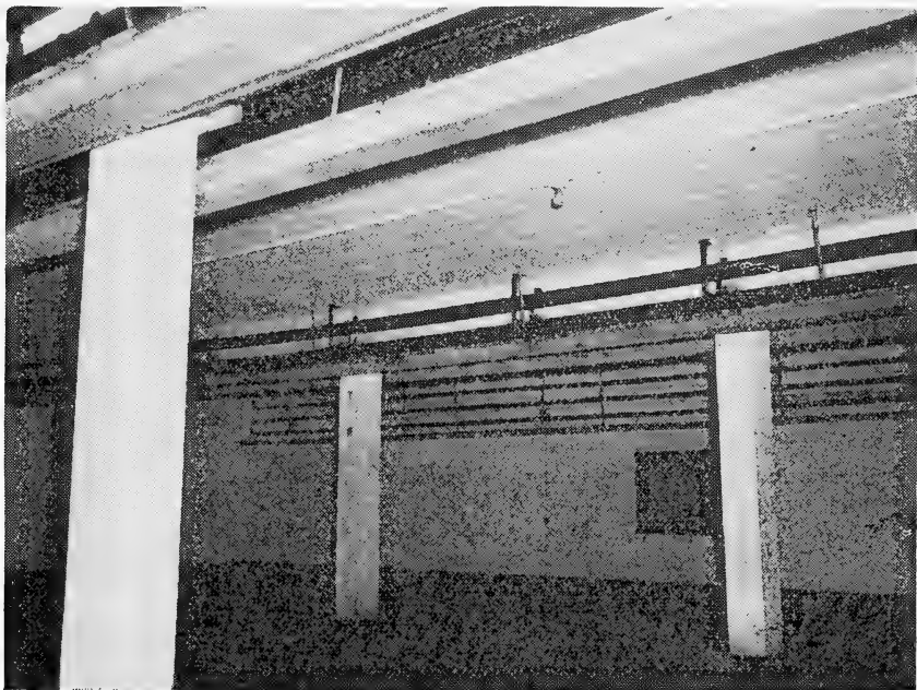
FIGURE 4.—Cold-storage room piped for direct-expansion system, with gutters suspended beneath pipes over the space to be occupied by fruit.
