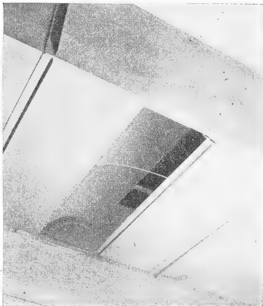
FIGURE 15.—View from below of a duct opening near the fan room in a reverse air system. The opening is narrow, and an internal deflector vane, or scoop, is used to divert the proper quantity of air to this part of the room.
