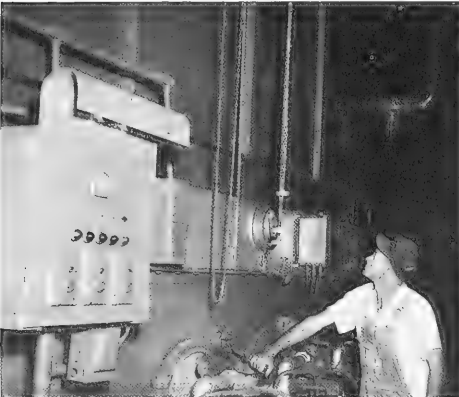
Fig. 1 - Steam power is needed in fishery byproducts plant. It is used to cook the raw fish, evaporate the water in making condensed fish solubles, and in many plants, for heating the meal dryers. This is a scene in a plant at Moss Point, Miss.
