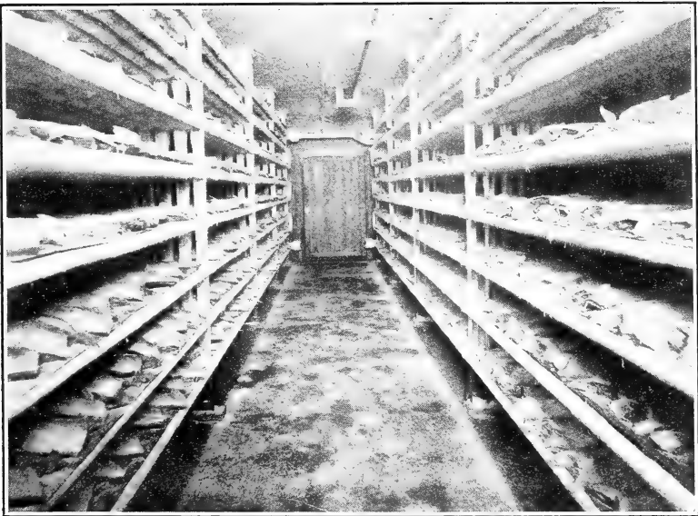
FIG. 2.—SHARP FREEZER ROOM.
