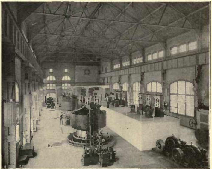
NIAGARA POWER-HOUSE (INTERIOR)
