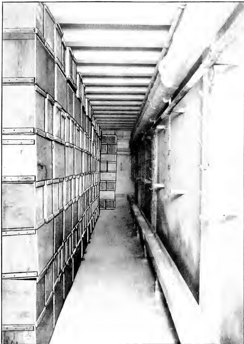
COLD-STORAGE ROOM, SHOWING BRINE COILS AND STACKS OF STORAGE-PACKED EGGS. CAPACITY, 4,000 CASES, OR 1,440,000 EGGS.
