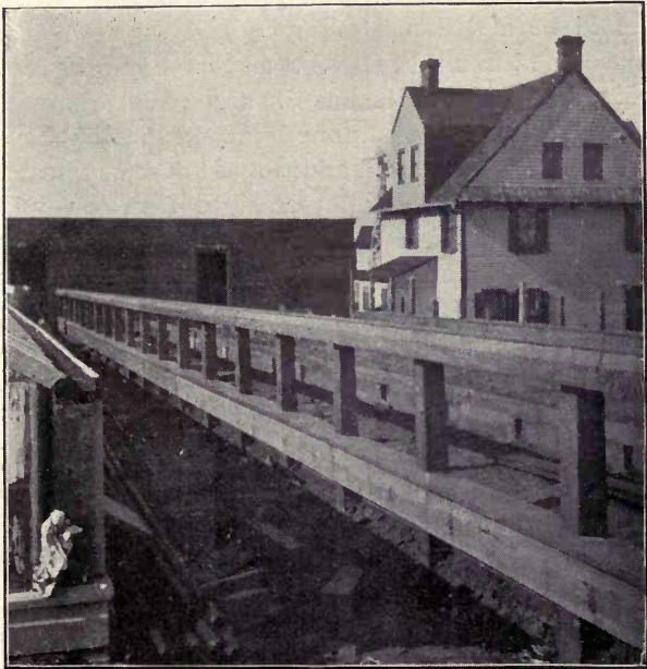
24.—Constructing house twenty-four feet wide; third step, running gutters and notching plate around posts.
