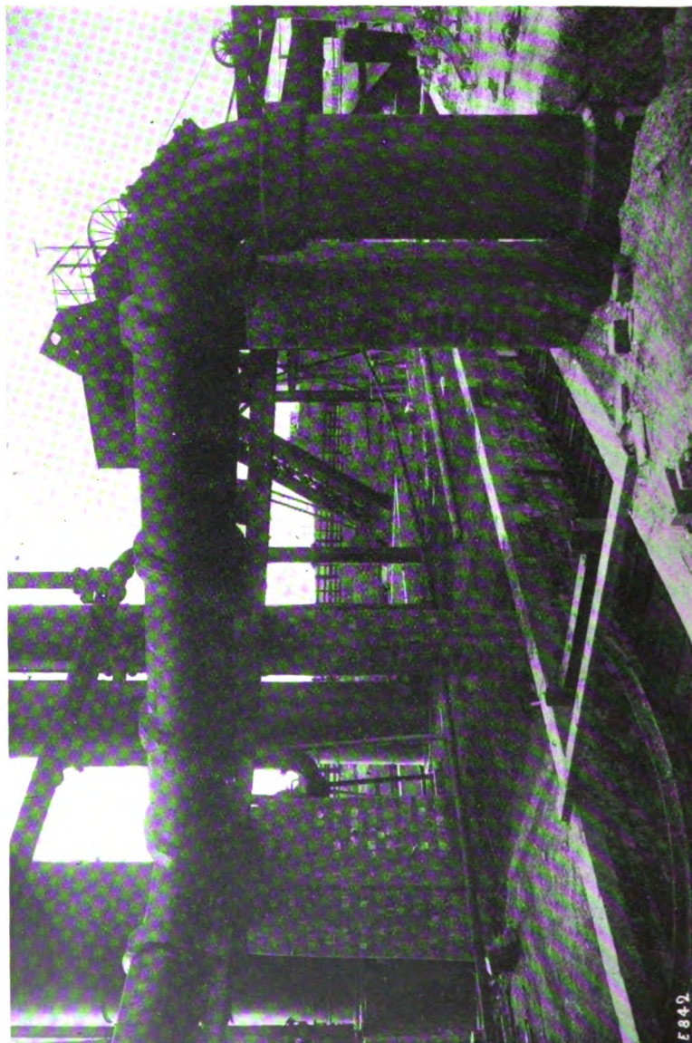
A 24-IN. REINFORCED CONCRETE GAS MAIN, SHOWING BEND IN CAST IRON WITH MANHOLE.
