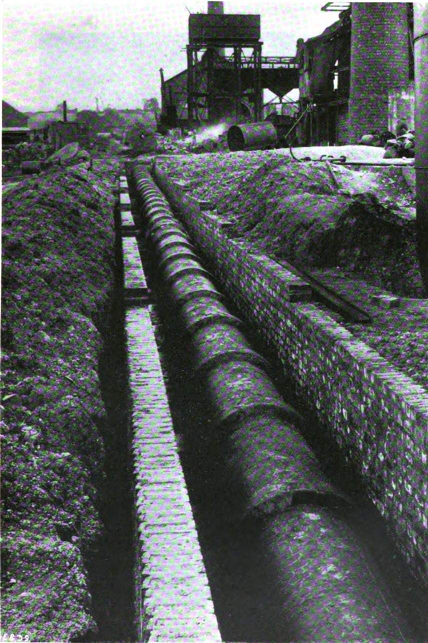
A 24-IN. REINFORCED CONCRETE GAS MAIN.
