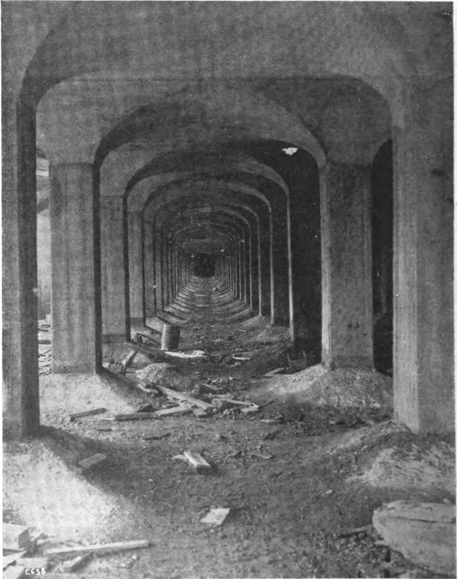
FIG. 9. View under Groined Arches. A LARGE FILTRATION PLANT AT ST. LOUIS, U.S.A.
