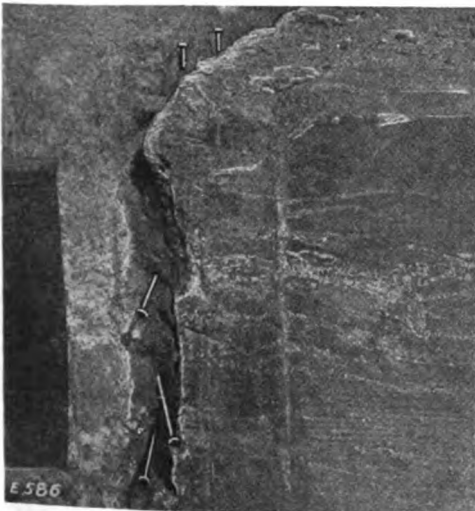
Fig. 7. Spikes Driven into Laitance at Top of Column. WATER THE CHIEF FACTOR IN THE MAKING OF GOOD CONCRETE.
