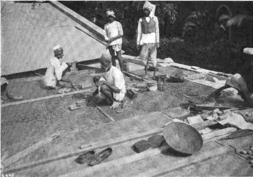
Fig. 2. A Test Roof Cover in course of construction in Bombay. REINFORCED CONCRETE ROOFS IN INDIA.
