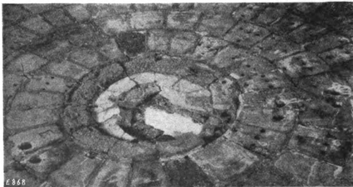
FIG. 6. VIEW SHOWING FRACTURE DUE TO IMPACT AT CENTRE OF DOME.
