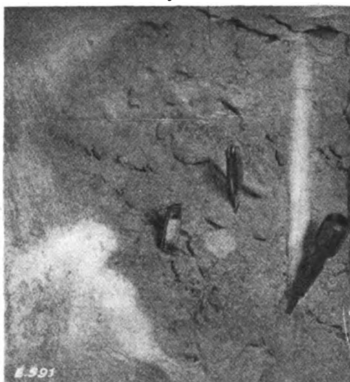
Fig. 3. The Result of Neglect in Precautions in Making Concrete.
