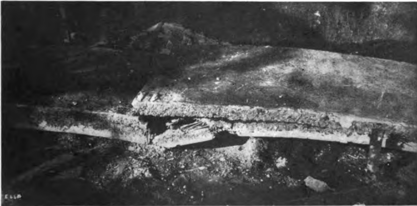
Fig. 4. A Section of Roofing Slabs constructed as a test. REINFORCED CONCRETE ROOFS IN INDIA.
