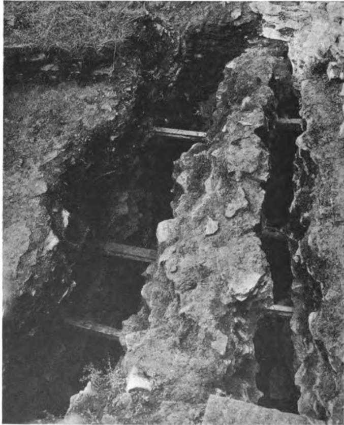
RICHMOND CASTLE. Cracks between East Curtain and Fallen Tower.
