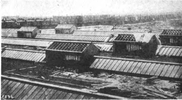
FIG. 8. CAR BARN OF THE PHILADELPHIA RAPID TRANSIT CO., SHOWING CONSTRUCTION OF REINFORCED CONCRETE SKYLIGHTS.
