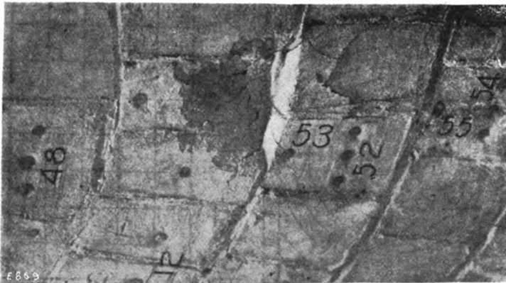
FIG. 8. VIEW SHOWING FRACTURE DUE TO IMPACT ON UNPROTECTED SURFACE.
