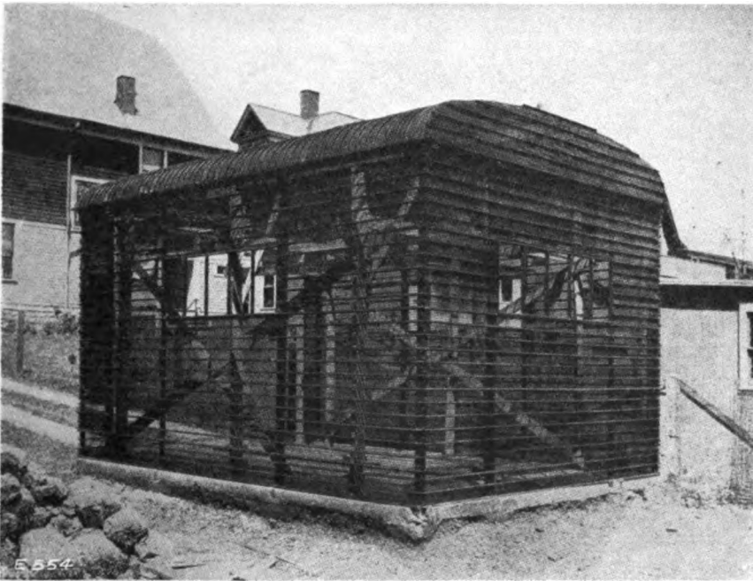
Fig. 7. Metal Lath Framework to be covered with Stucco or Cement Plaster. SMALL CONCRETE GARAGES.
