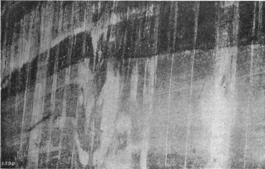
Fig. 2. The concrete in this wall was poured with excess of water, and shows thick bands of laitance. WATER THE CHIEF FACTOR IN THE MAKING OF GOOD CONCRETE.
