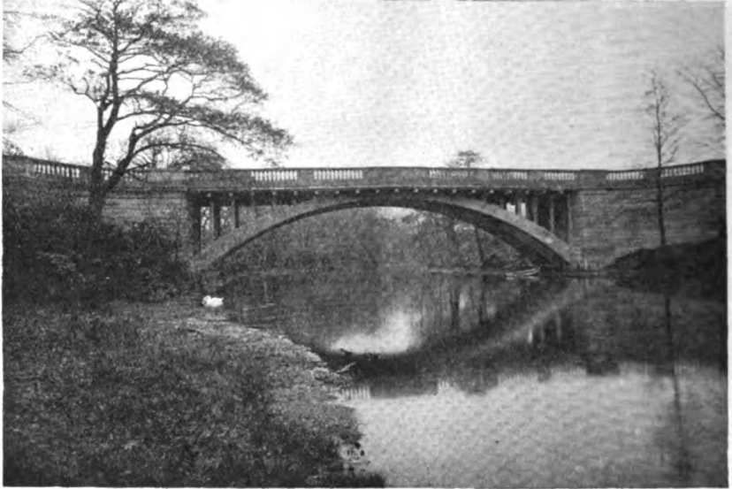
Bridge over Lymm Dam, Cheshire, for the Lymm Estates Co. Architects: Messrs. Wm. & Segar Owen Reinforced entirely on B.R.C. System.
