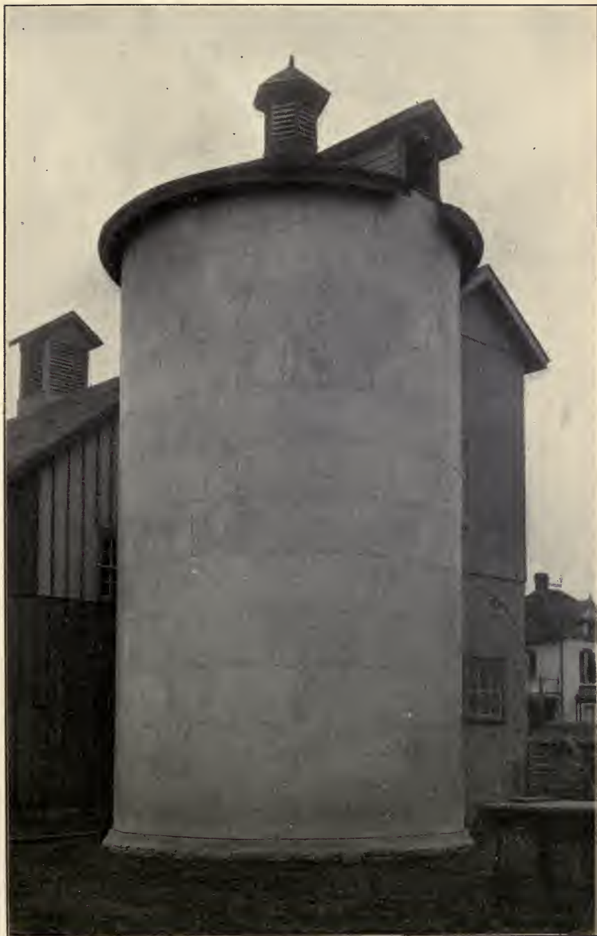
CUT 25.—SAME CONSTRUCTION AS SHOWN IN CUT 22; SHEETED WITH HALF-INCH LUMBER TO A HEIGHT OF SIX FEET AND COVERED WITH GALVANIZED IRON. AN EXPENSIVE COVERING BUT DURABLE AND SAVES PAINTING
