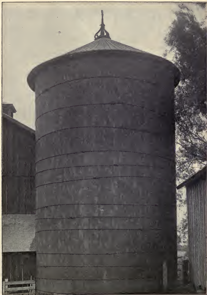
CUT 33.—STAVE SILO 20 FEET IN DIAMETER AND 34 FEET DEEP; CAPACITY 224 TONS. THE STAVES HAVE SHRUNK WHEN EMPTY ALLOWING HOOPS TO DROP FROM ORIGINAL POSITION.
