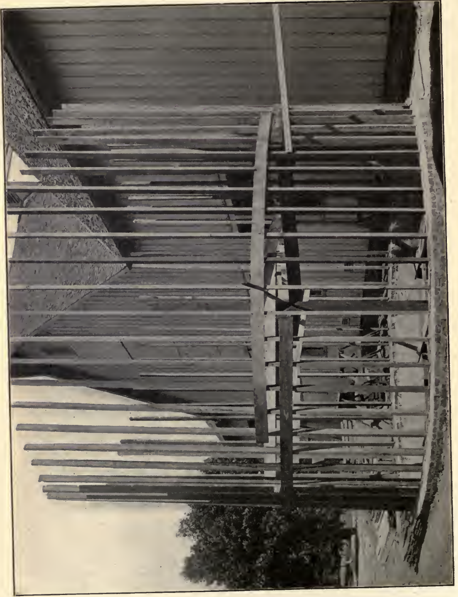
CUT 12.—2X4 STUDS SET ON SILL AND PLUMBED TO HEIGHT OF SIX FEET.
