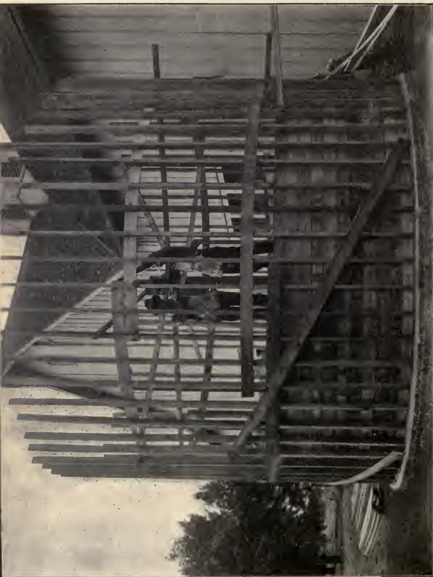
CUT 13.—SILO CEILED ON INSIDE TO HEIGHT OF SIX FEET. PLUMBING SECOND SIX FEET OF STUDS.
