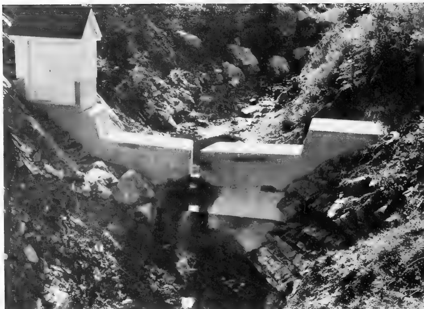
Figure 7.--Modified Venturii-trapezoidal flume in a broad-crested weir section constructed in the late 1930's on the Davis County Experimental Watershed.
