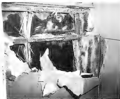
Damage to structural timbers (Wallboard removed to expose damage)
