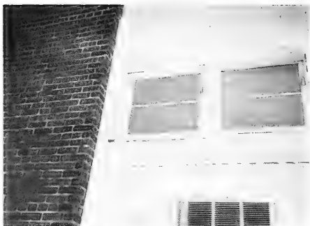
Note tunnels around window frame
