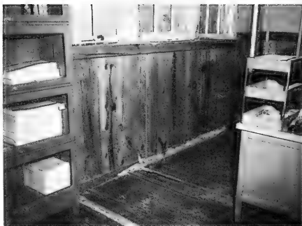
Damage to floor and base of cabinet
