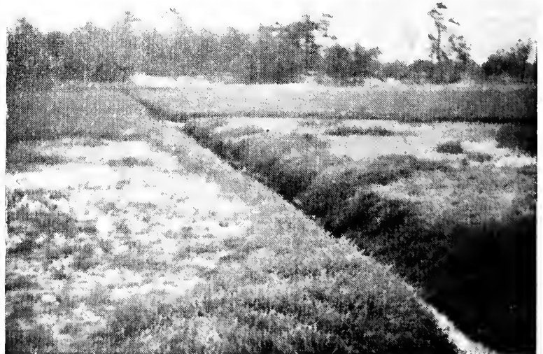
Top—Poor land drainage. The stake is at the end of a tile drain. There is a nine in fall in three feet yet water is standing on the surface at the right.
